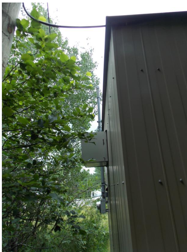
49 Shelter View (Electrical Service, AC unit)
