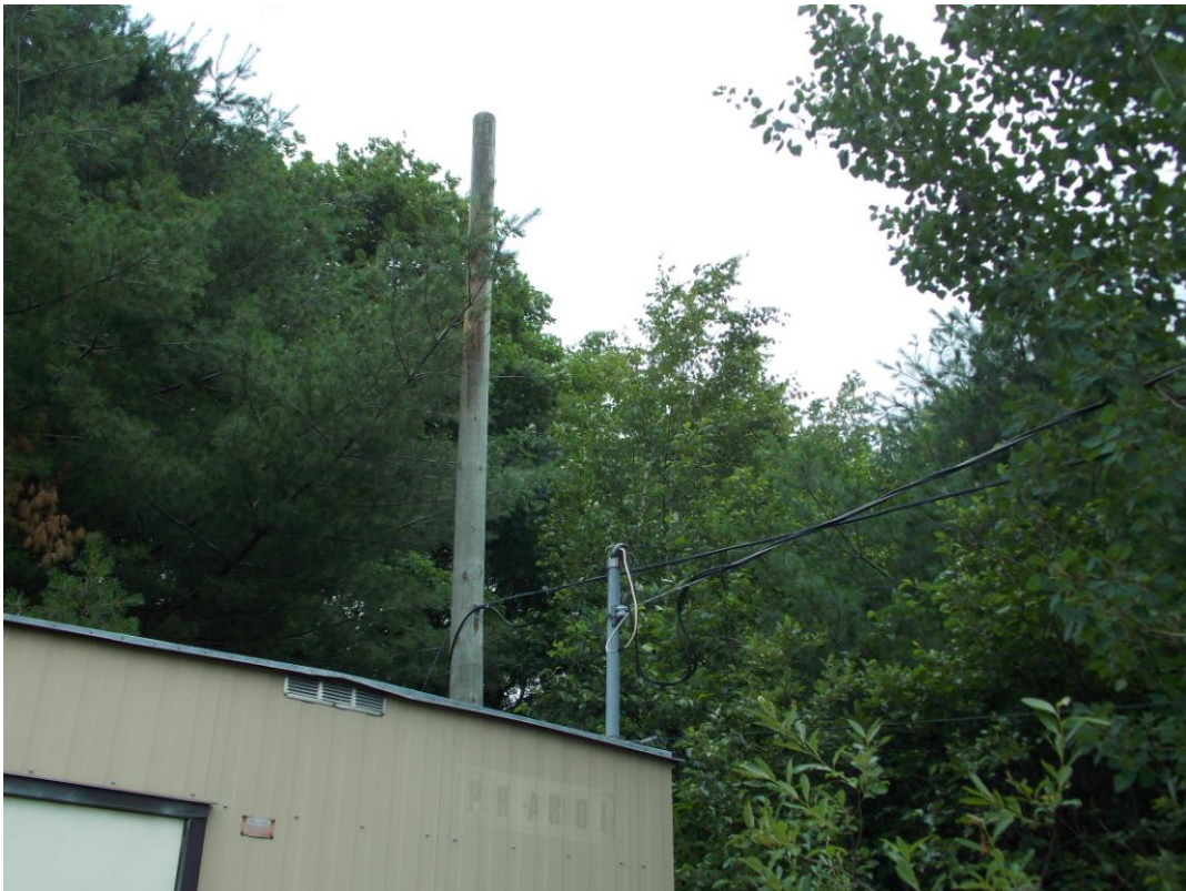
33 Electrical Service Entrance
