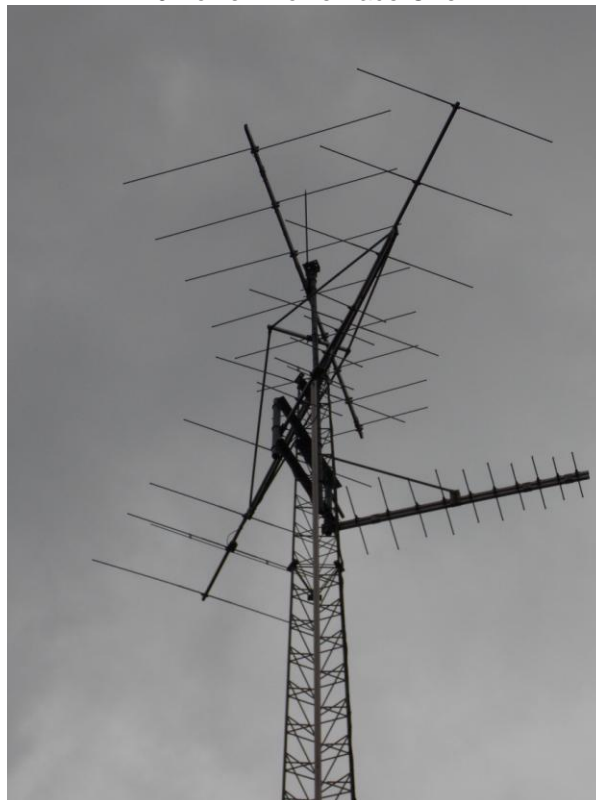
10 Antenna Configuration Face One
