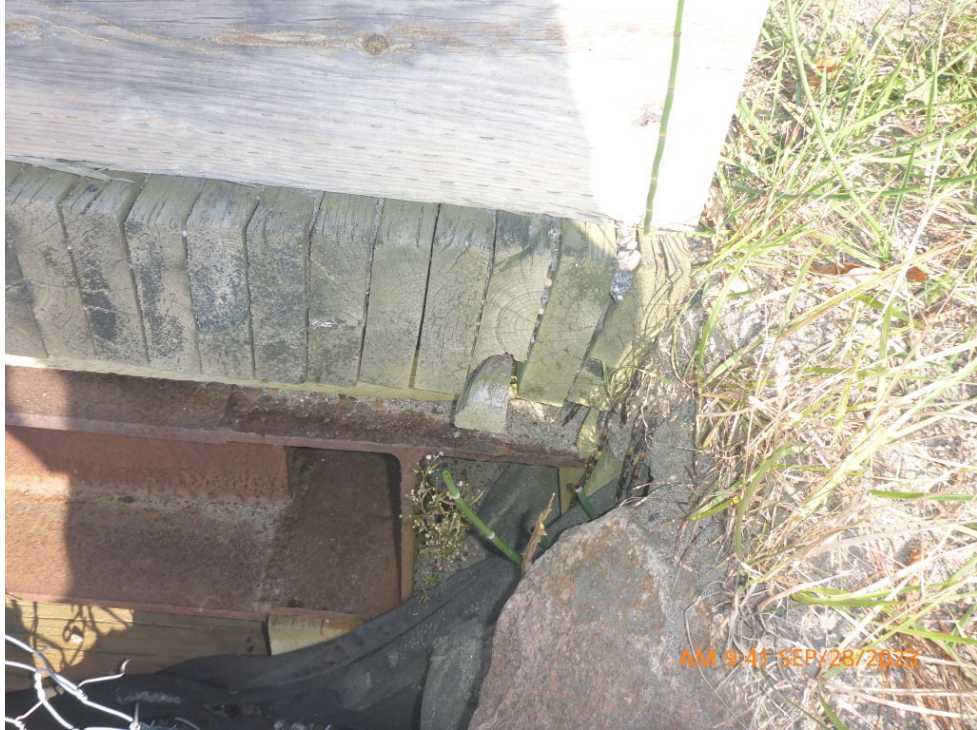
Comments: SEVERE SPLIT IN TIMBER DECK MEMBER EAST APPROACH
