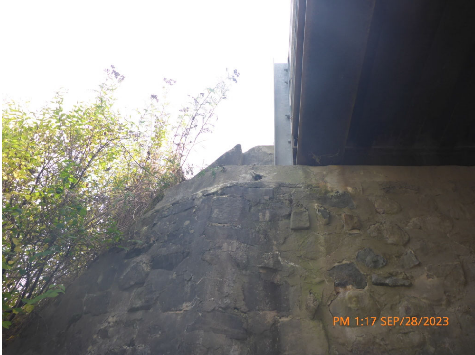
Comments: EFFLORESCENT STAINING SOUTH ABUTMENT CAP Path: P:\McKellar\2023\P1080223.jpg
