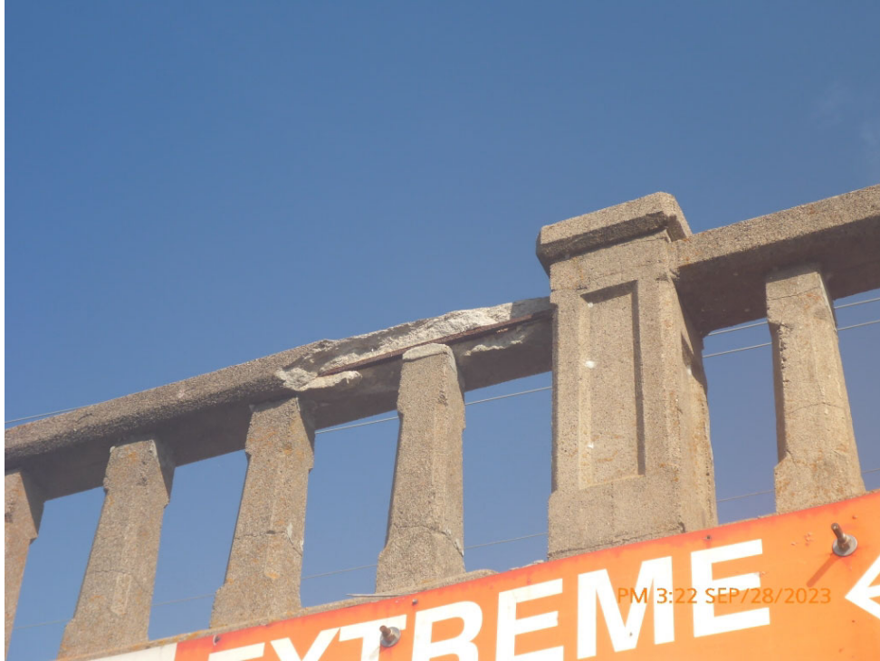
Comments: SPALLING OF BALUSTRADE RAILING Path: P:\McKellar\2023\P1080295.jpg
