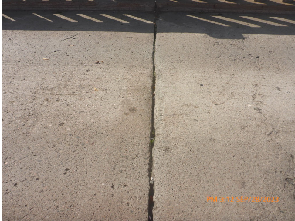
Comments: GAP AT MIDSPAN OF DECK
