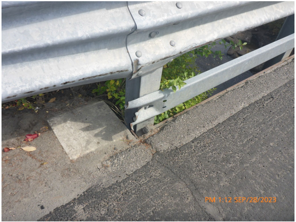
Comments: COLLISION DAMAGE GUIDE RAIL C-CHANNEL Path: P:\McKellar\2023\P1080212.jpg
