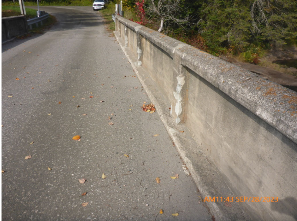
Comments: MEDIUM SCALING ALONG CURB LINE
