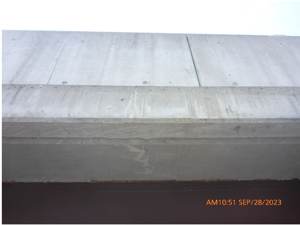
Comments: NARROW STAINED CRACK EXTERIOR SOFFIT Path: P:\McKellar\2023\P1080147.jpg
