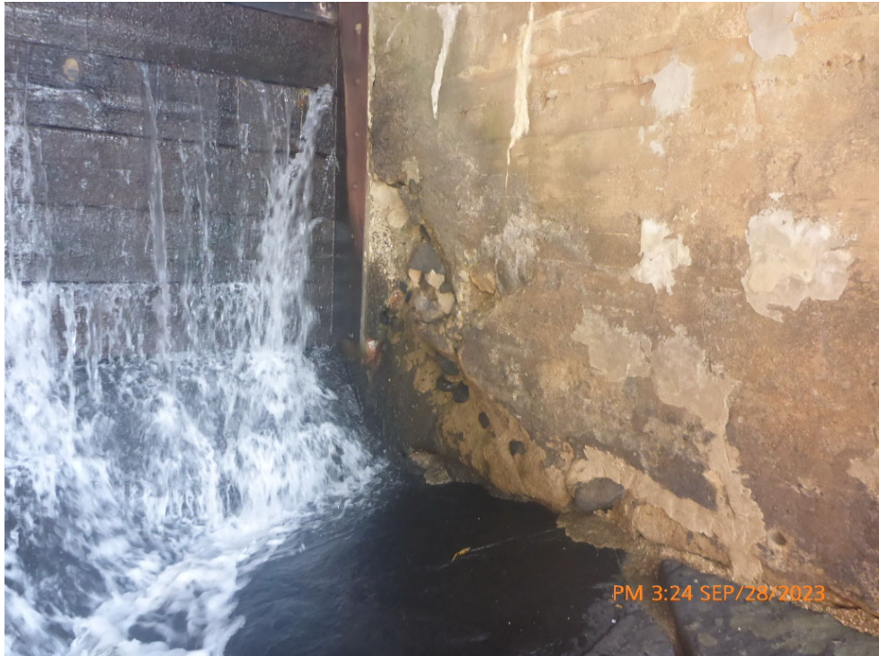
Comments: SEVERE SCOURING OF SOUTH ABUTMENT
