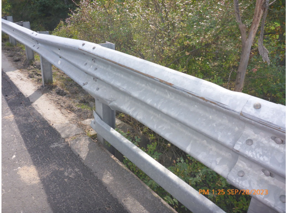
Comments: MINOR COLLISION DAMAGE THRIE BEAM GUIDE RAIL Path: P:\McKellar\2023\P1080233.jpg
