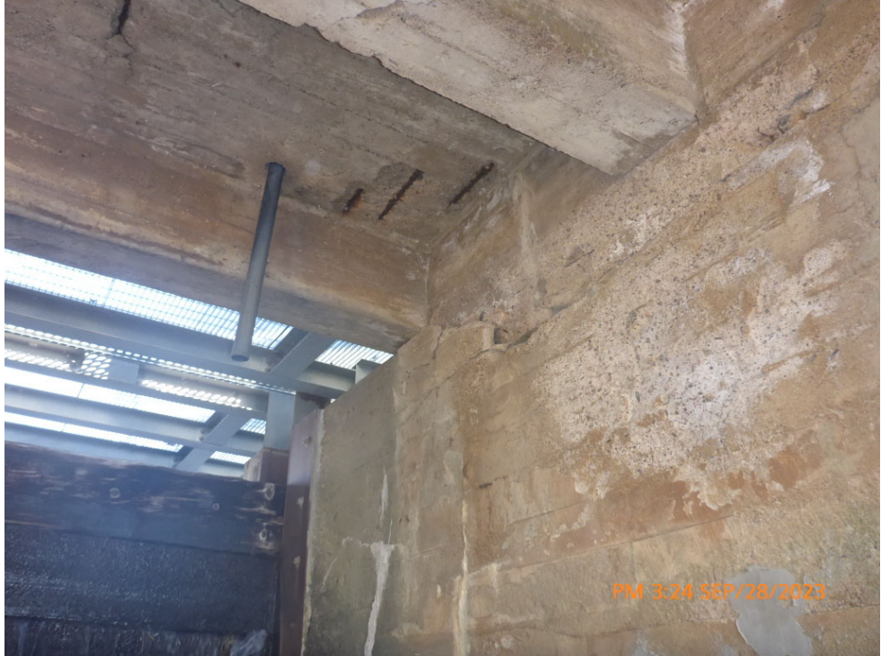
Comments: SEVERE DELAMINATIONS SOUTH ABUTMENT Path: P:\McKellar\2023\P1080300.jpg
