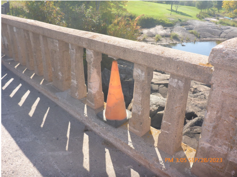
Comments: MISSING BALUSTRADE WEST RAILING
