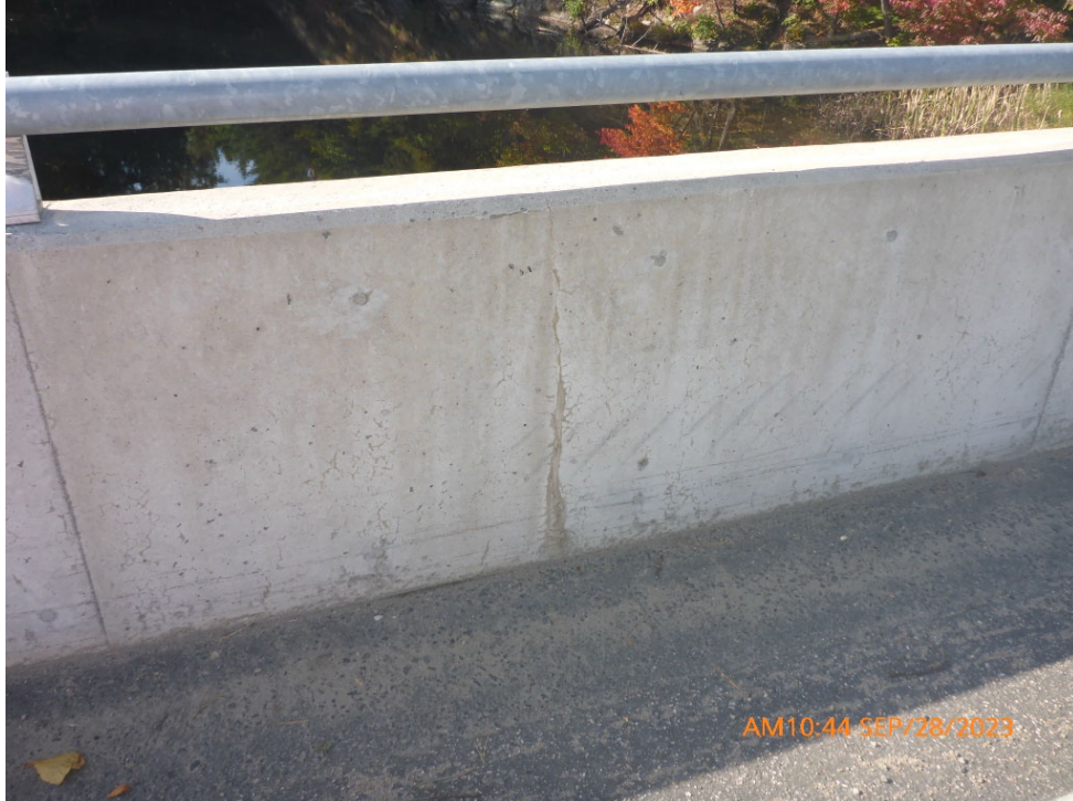
Comments: NARROW STAINED CRACK IN INTERIOR PARAPET WALL
