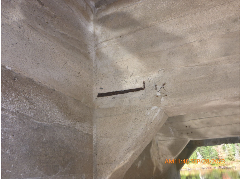
Comments: SPALLING OF T-BEAM GIRDER
