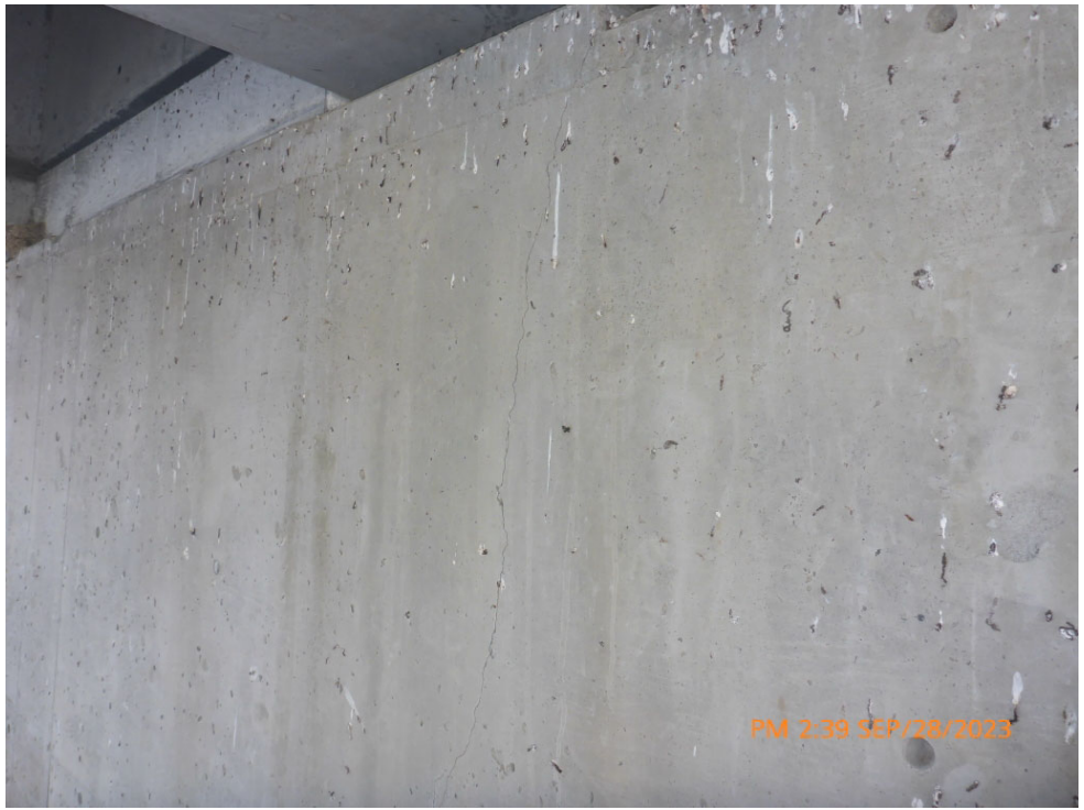
Comments: MEDIUM VERTICAL CRACK SOUTH ABUTMENT
