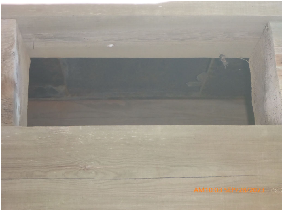
Comments: SEVERE FLAKING OF STEEL BALLAST WALL WEST ABUTMENT Path: P:\McKellar\2023\P1080125.jpg
