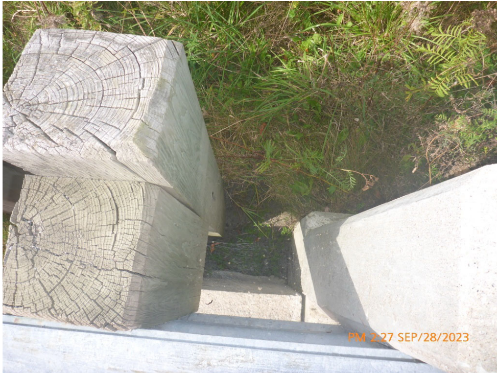
Comments: EROSION IN SOUTHWEST QUADRANT
