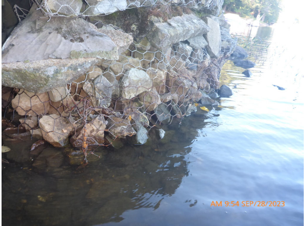
Comments: LOSS OF ROCK FILL GABION BASKET RETAINING WALL
