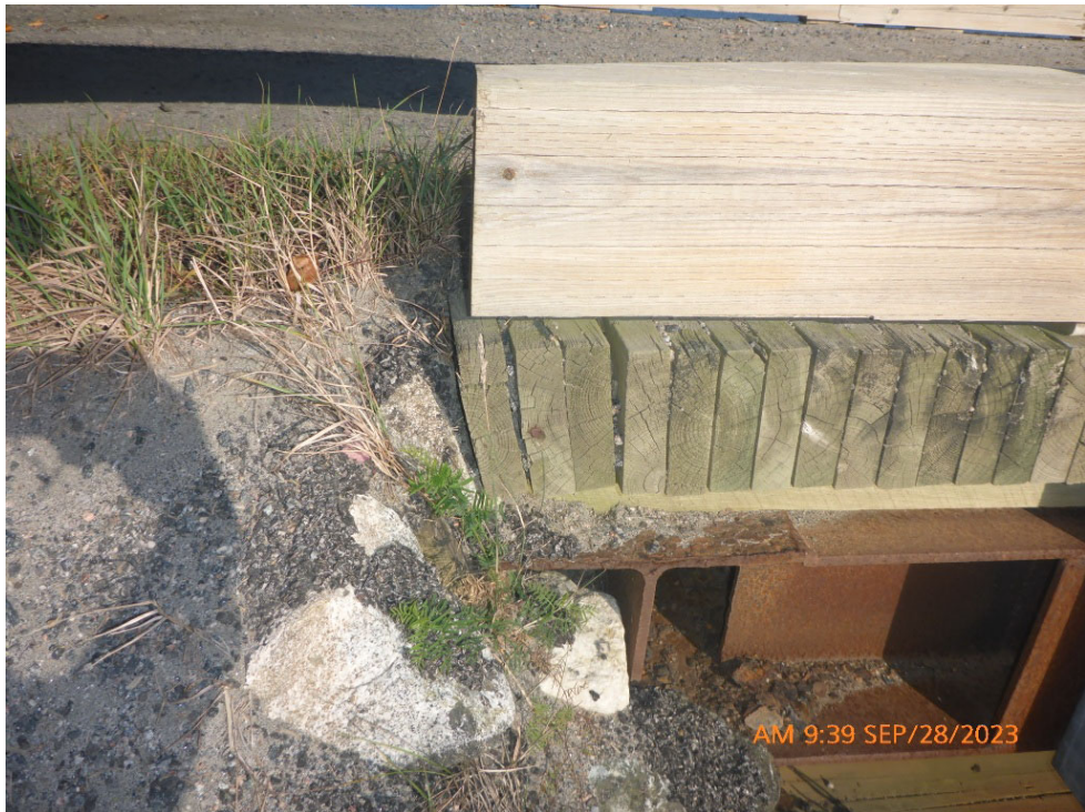
Comments: ROTATION OF TIMBER DECK MEMBERS EAST APPROACH
