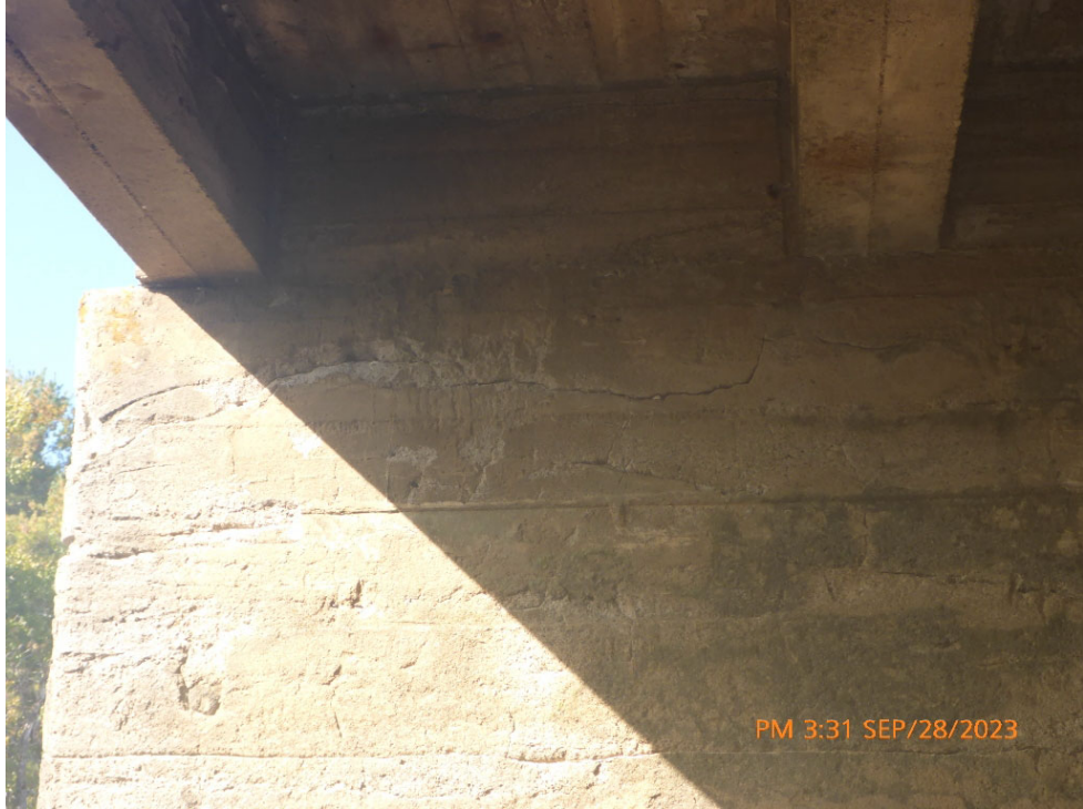
Comments: WIDE HORIZONTAL CRACK IN PIER
