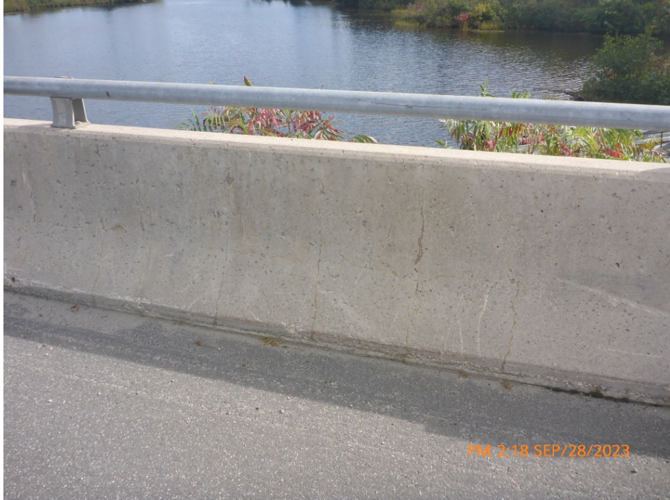
Comments: NARROW STAINED CRACKS INTERIOR PARAPET WALL
