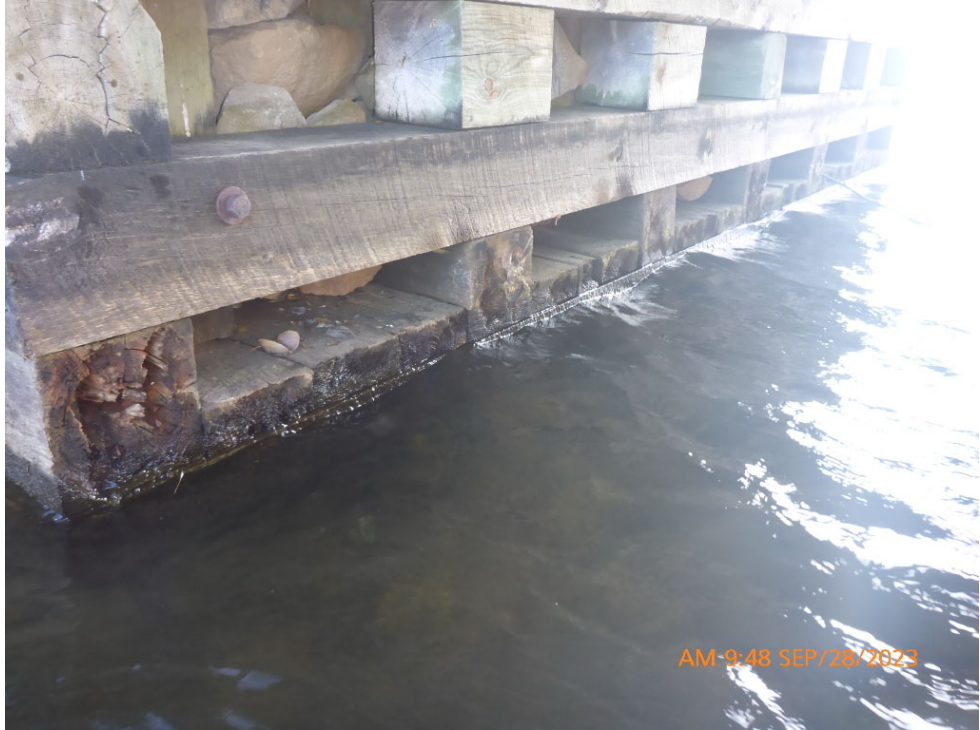
Comments: MEDIUM ROT OF TIMBER CRIB MEMBERS EAST ABUTMENT
