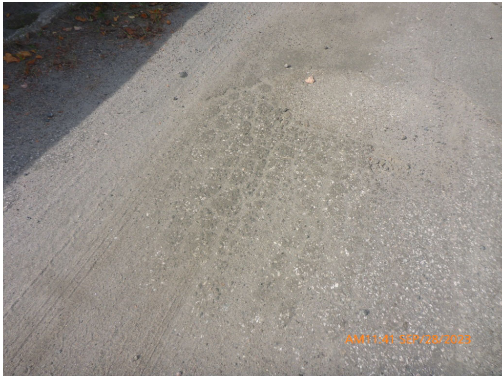
Comments: SEVERE MAP CRACKING APPROACH WEARING SURFACE Path: P:\McKellar\2023\P1080158.jpg
