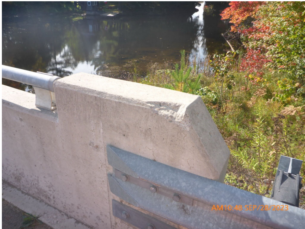
Comments: ABRASION PARAPET END POST
