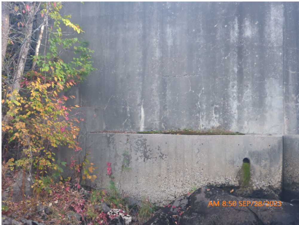
Comments: NARROW STAINED CRACK IN WINGWALL
