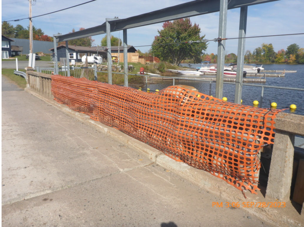
Comments: MISSING BALUSTRADES ON EAST RAILING
