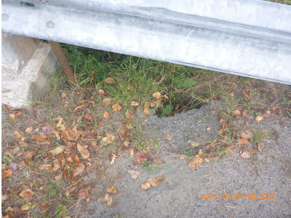
Comments: SEVERE EROSION OF EMBANKMENT NE QUADRANT
