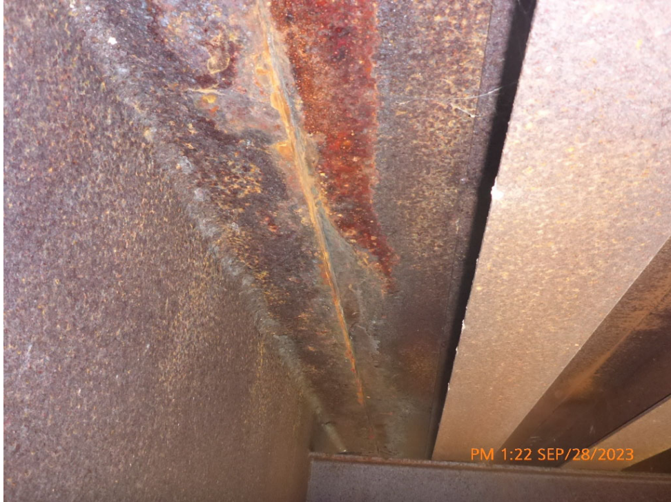
Comments: MEDIUM FLAKING OF STEEL GIRDER BOTTOM FLANGE Path: P:\McKellar\2023\P1080232.jpg
