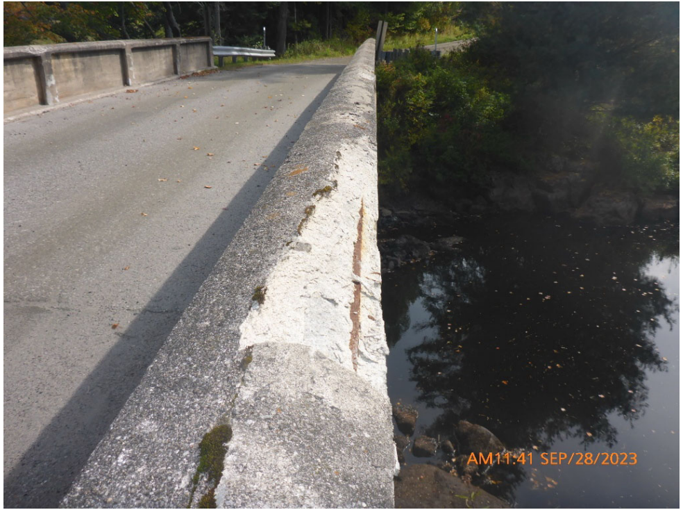
Comments: SEVERE SPALL BARRIER WALL
