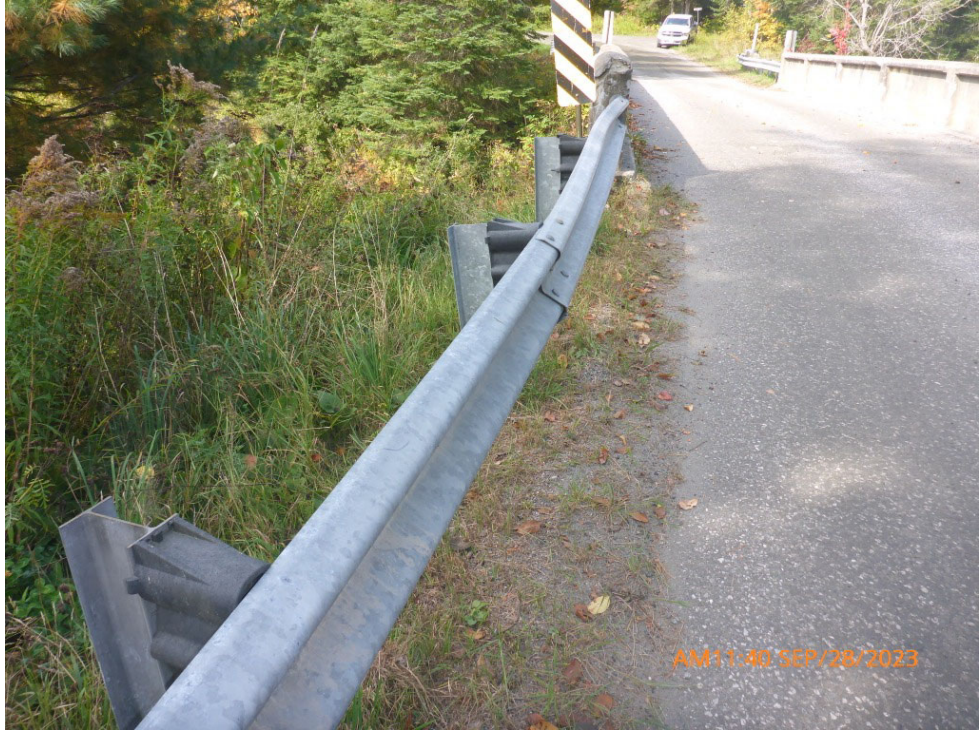
Comments: MINOR COLLISION DAMAGE GUIDE RAIL Path: P:\McKellar\2023\P1080157.jpg
