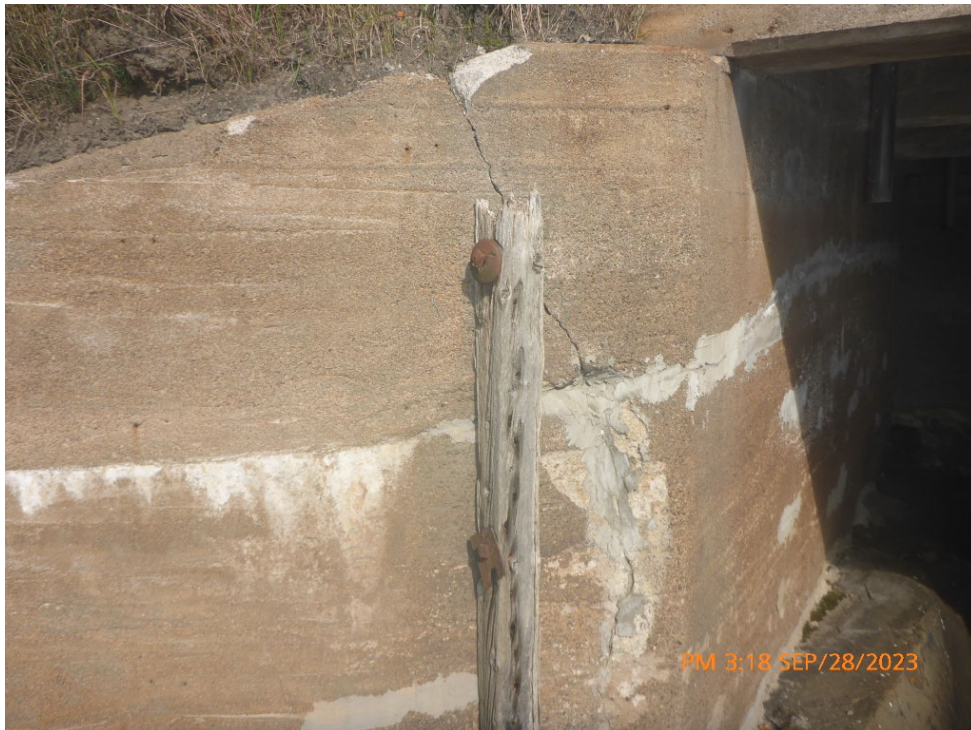
Comments: WIDE CRACK IN NORTHWEST WINGWALL Path: P:\McKellar\2023\P1080283.jpg
