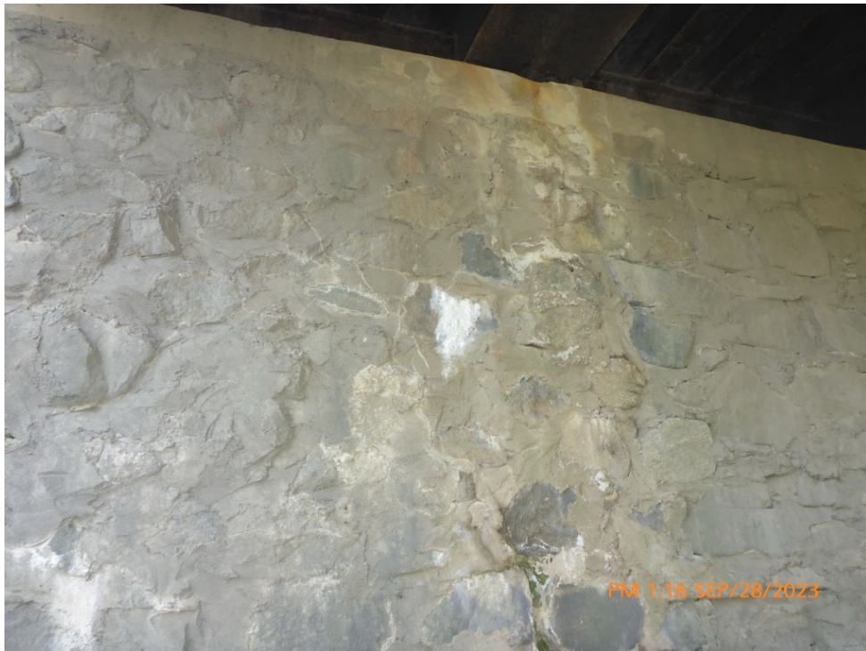
Comments: EFFLORESCENT STAINING SOUTH ABUTMENT Path: P:\McKellar\2023\P1080222.jpg
