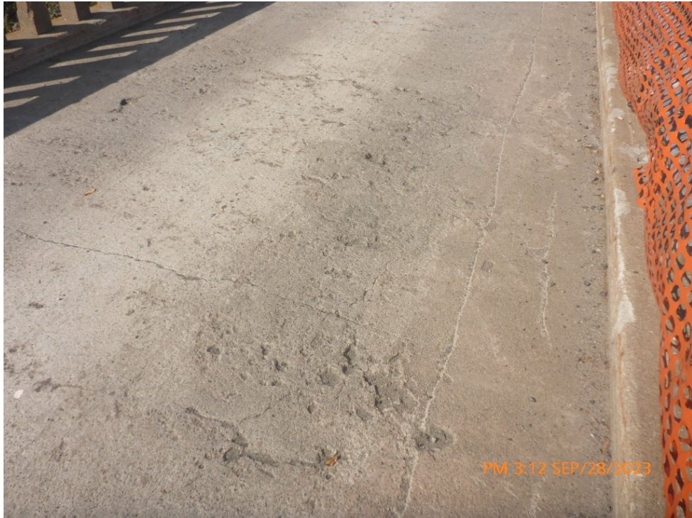
Comments: SEVERE SCALING OF CONCRETE DECK
