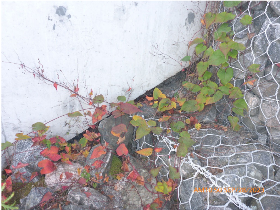
Comments: MODERATE UNDERMINING BELOW WINGWALL
