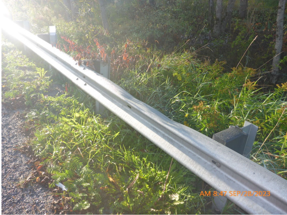
Comments: MINOR COLLISION DAMAGE GUIDE RAIL Path: P:\McKellar\2023\P1080084.jpg
