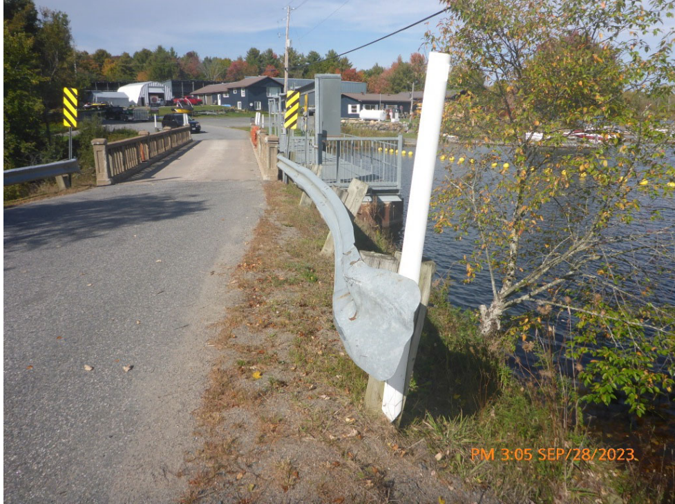
Comments: OUTWARD ROTATION OF APPROACH GUIDE RAIL SOUTHEAST QUADRANT
