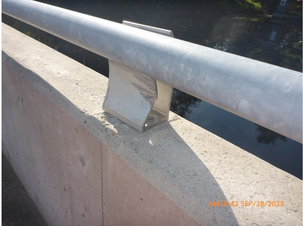
Comments: COLLISION DAMAGE PARAPET HAND RAILING Path: P:\McKellar\2023\P1080133.jpg
