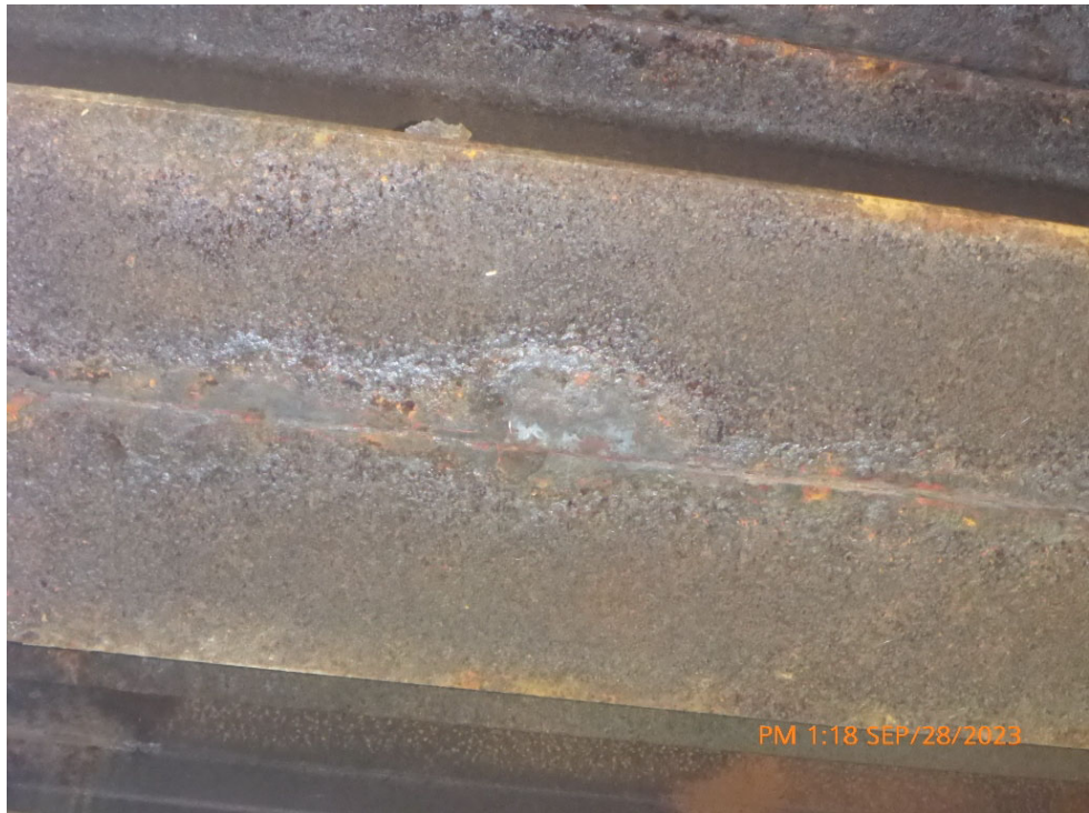
Comments: LIGHT FLAKING OF PATINA GIRDER
