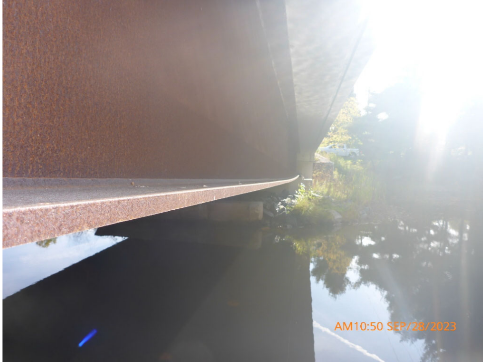
Comments: REVERSE CAMBER ON EXTERIOR GIRDER Path: P:\McKellar\2023\P1080143.jpg
