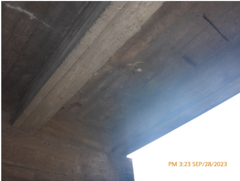
Comments: SEVERE DELAMINATIONS INTERIOR SOFFIT Path: P:\McKellar\2023\P1080296.jpg
