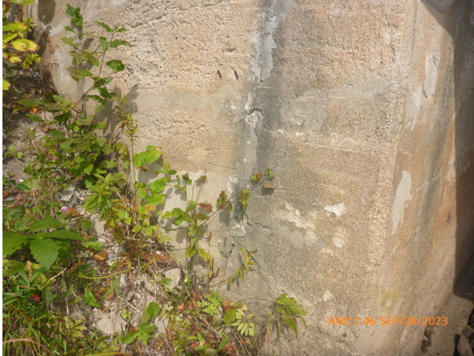
Comments: WIDE VERTICAL CRACK SOUTHWEST WINGWALL
