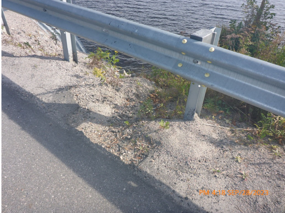
Comments: MINOR EROSION OF EMBANKMENT
