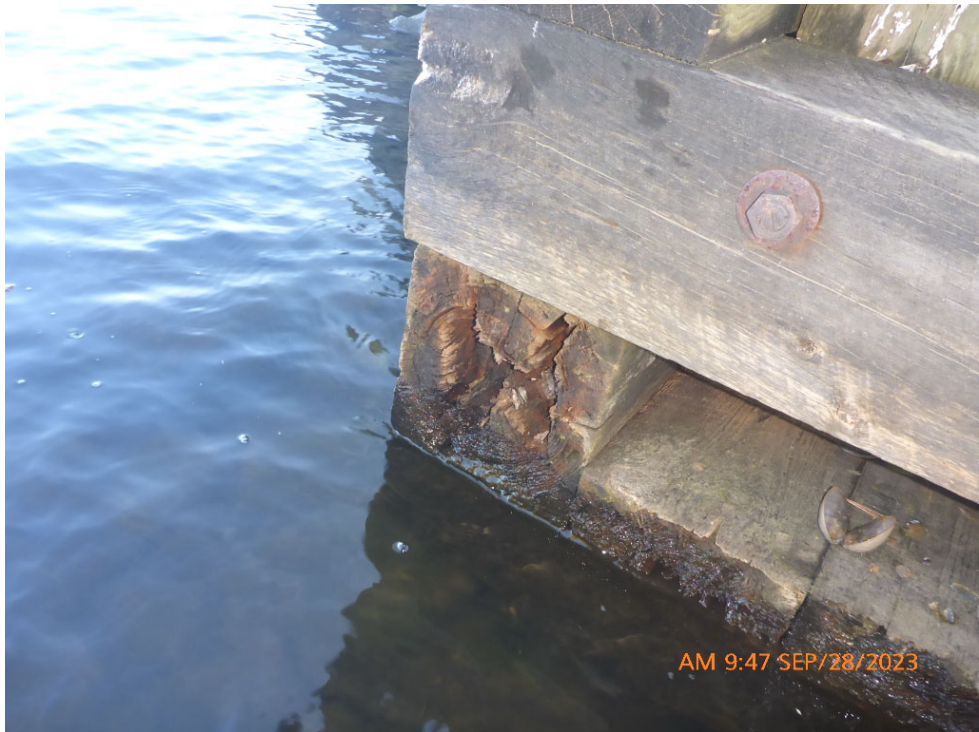
Comments: MEDIUM ROT OF TIMBER CRIB MEMBER
