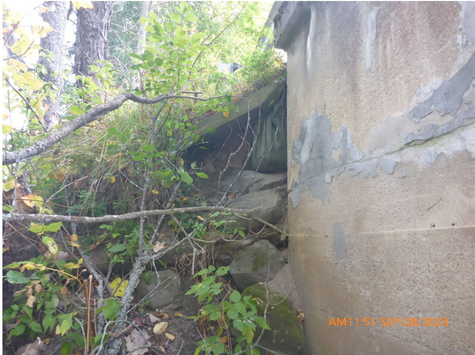
Comments: SEVERE EROSION NORTHEAST QUADRANT
