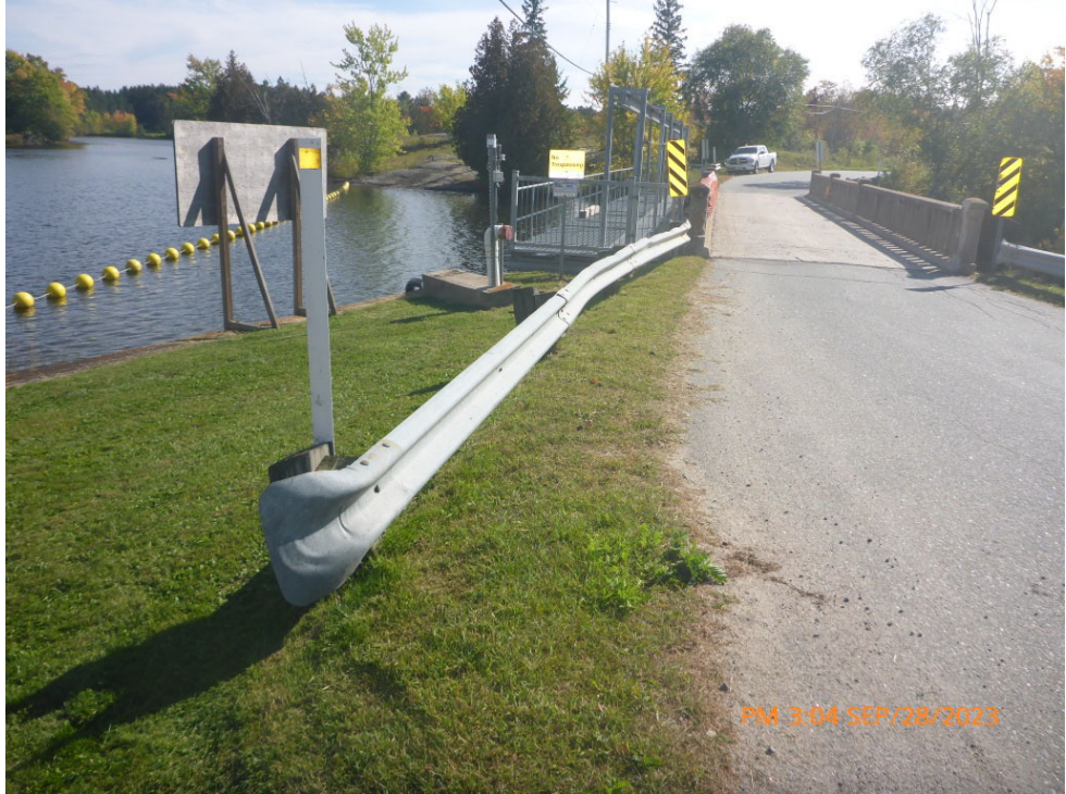
Comments: COLLISION DAMAGE TO NORTHEAST GUIDE RAIL
