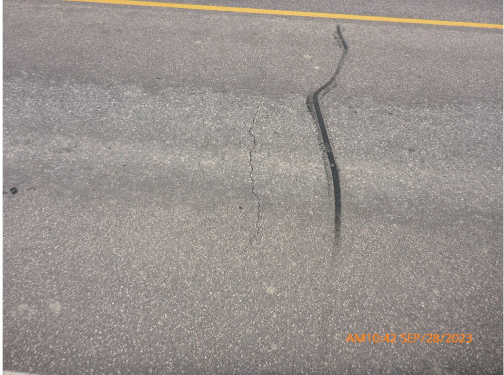
Comments: NARROW TRANSVERSE CRACK IN WEARING SURFACE Path: P:\McKellar\2023\P1080132.jpg
