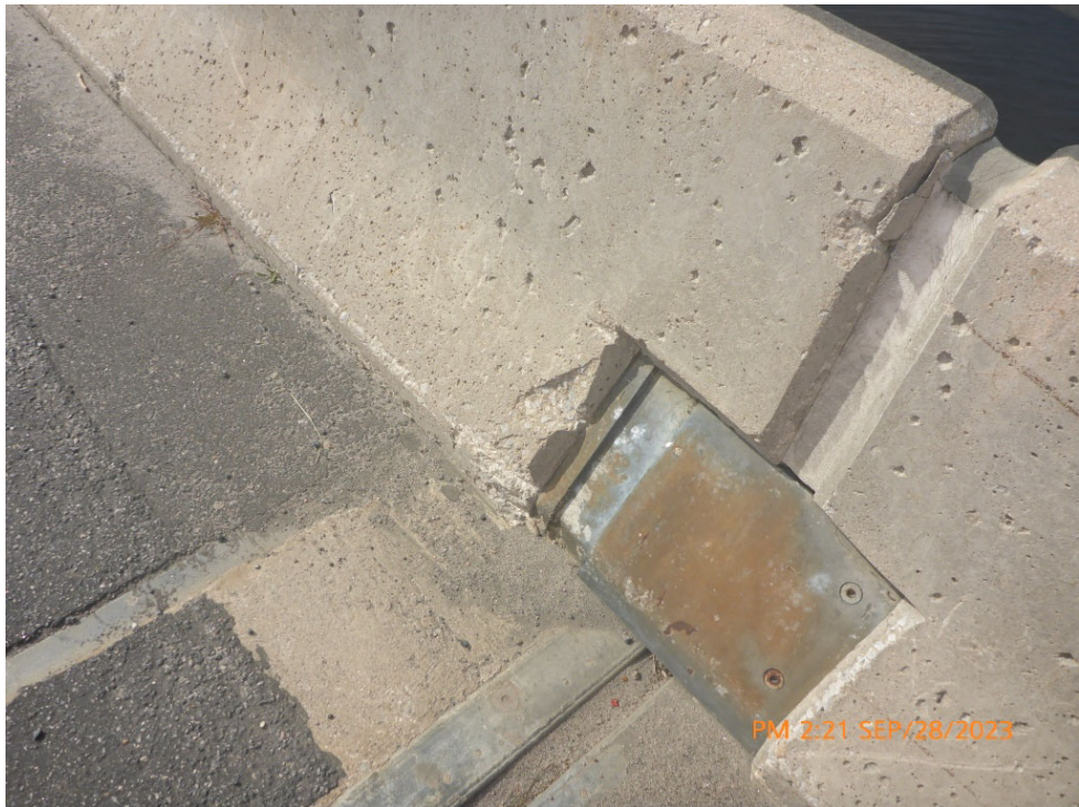
Comments: LIGHT ABRASION INTERIOR PARAPET WALL
