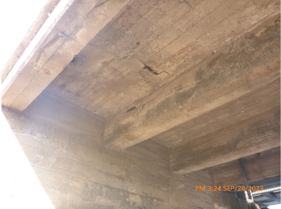
Comments: SEVERE DELAMINATIONS INTERIOR SOFFIT Path: P:\McKellar\2023\P1080298.jpg
