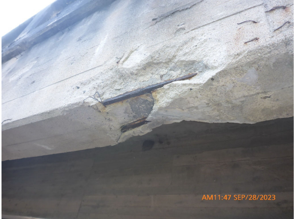
Comments: SEVERE SPALLING OF T-BEAM GIRDER Path: P:\McKellar\2023\P1080179.jpg
