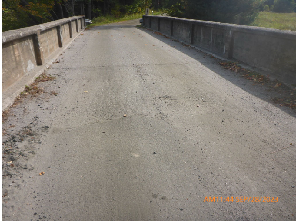
Comments: SETTLEMENT OF WEST APPROACH
