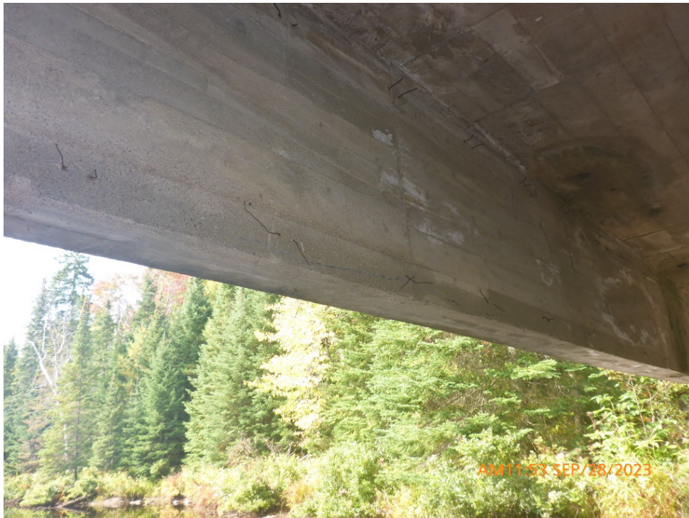
Comments: SEVERE DELAMINATION T-BEAM GIRDER
