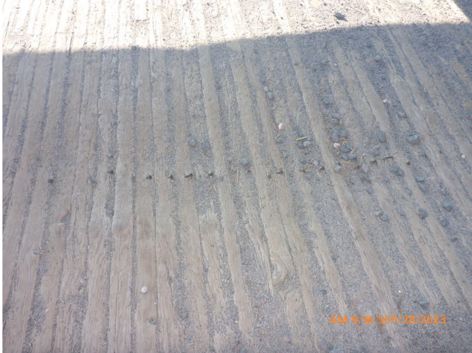
Comments: PROTRUDING NAILS IN TIMBER DECK MEMBERS
