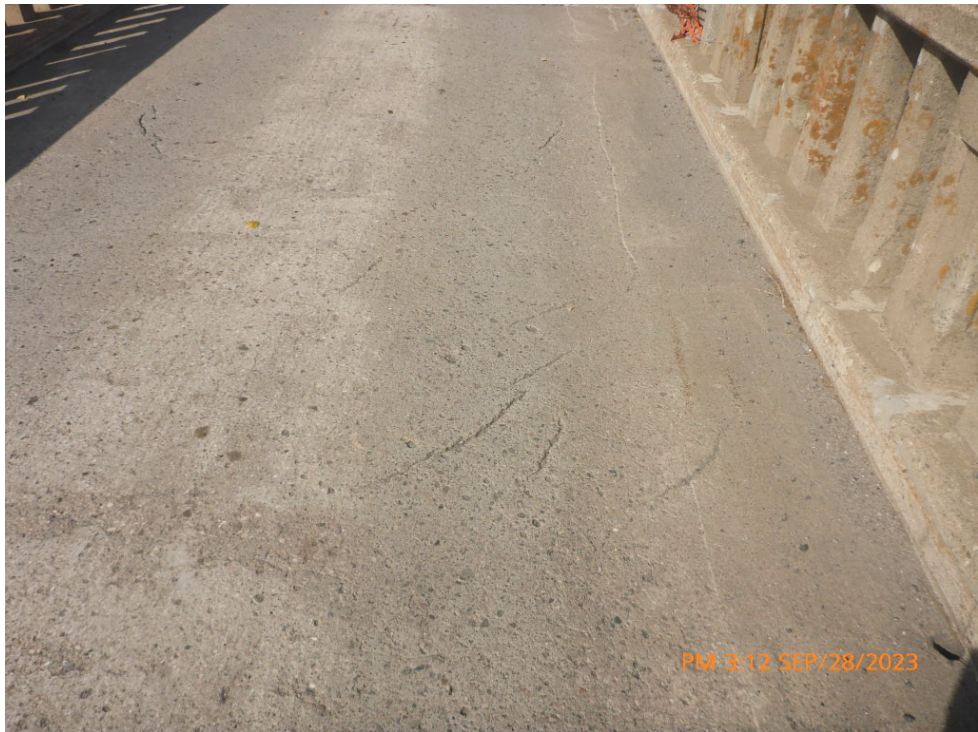
Comments: WIDE CRACKS IN CONCRETE DECK
