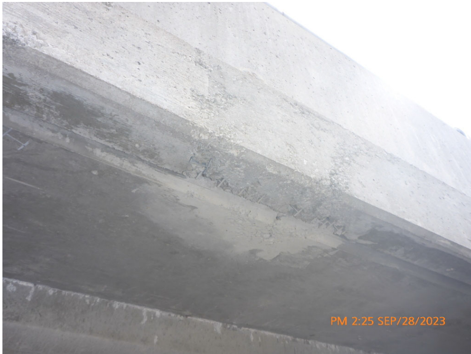
Comments: MEDIUM HONEYCOMBING EXTERIOR GIRDER
