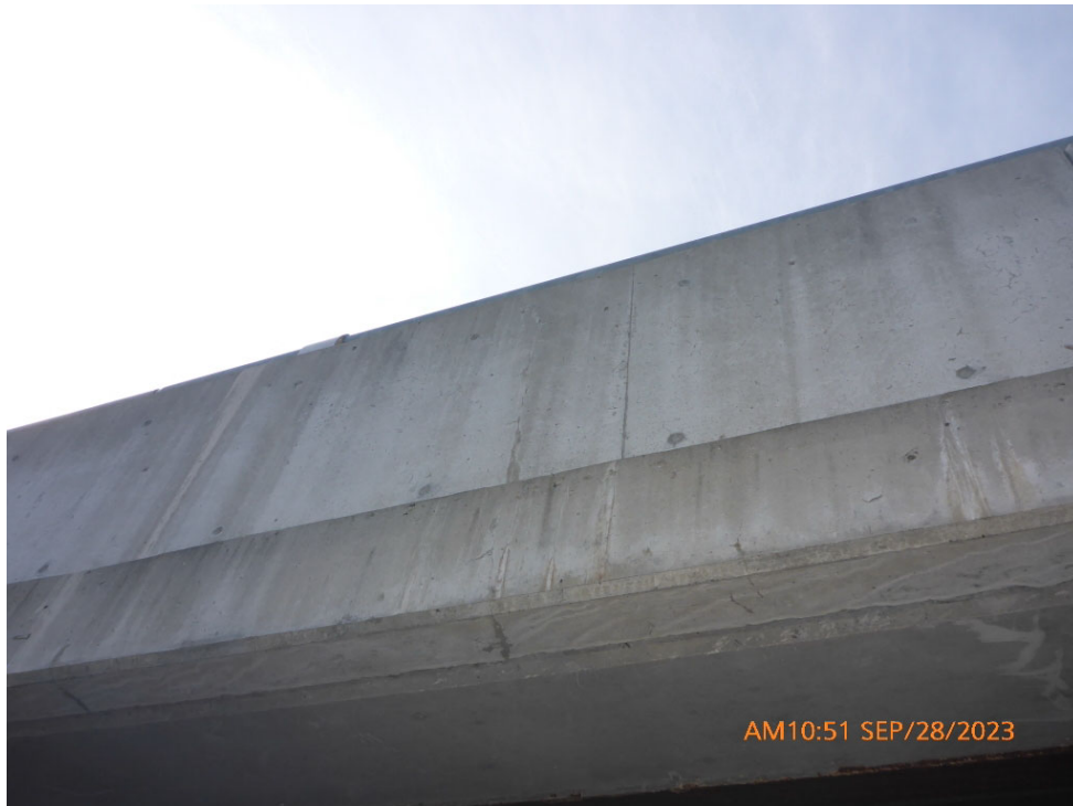
Comments: NARROW STAINED CRACK EXTERIOR PARAPET WALL Path: P:\McKellar\2023\P1080148.jpg
