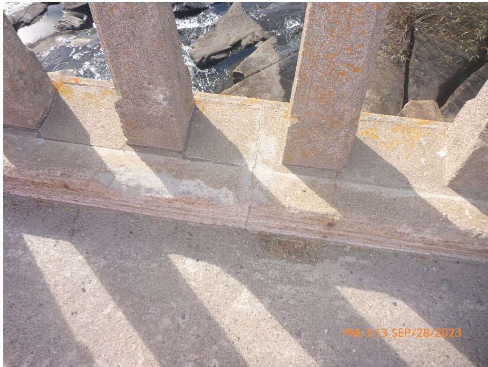
Comments: WIDE CRACK IN CONCRETE CURB
