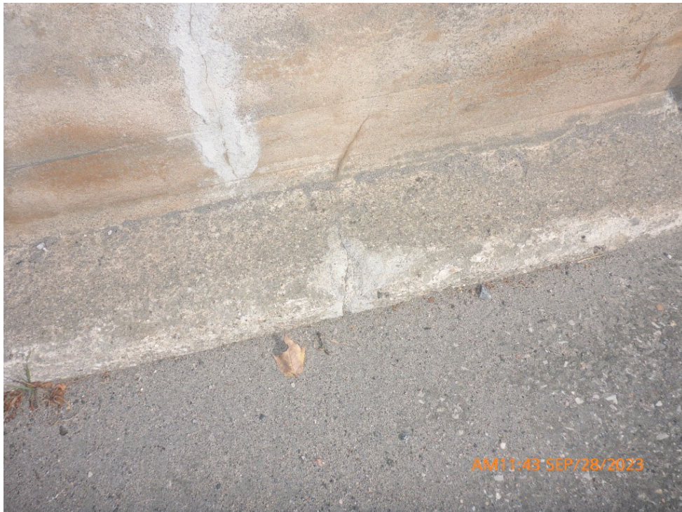
Comments: WIDE CRACK IN CONCRETE CURB
