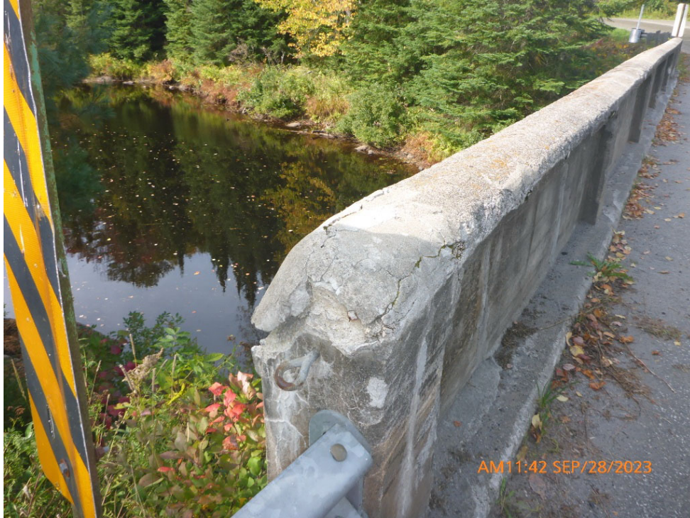
Comments: DEBONDED CONCRETE PATCH BARRIER WALL
