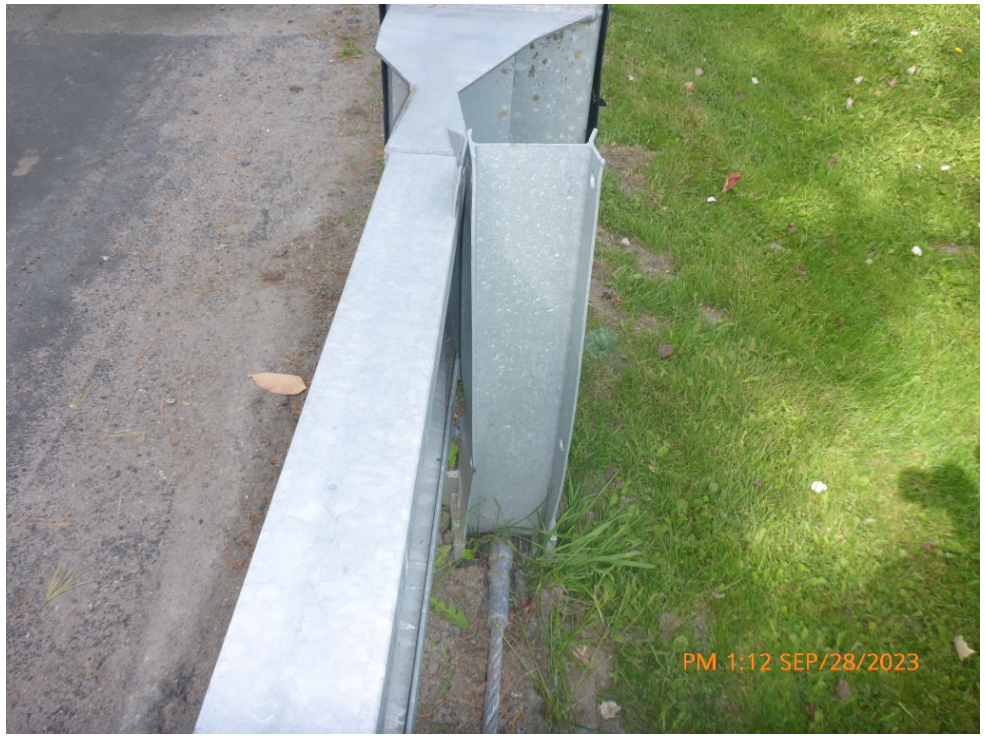
Comments: COLLISION DAMAGE NORTHEAST END TREATMENT POST Path: P:\McKellar\2023\P1080209.jpg
