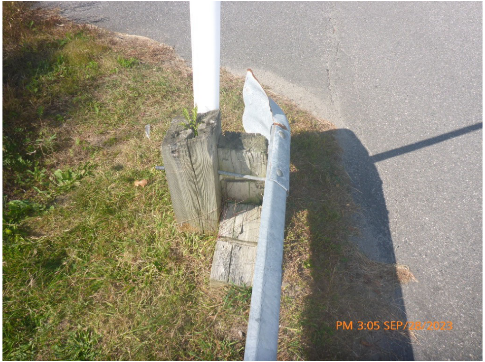
Comments: BROKEN OFFSET BLOCK
