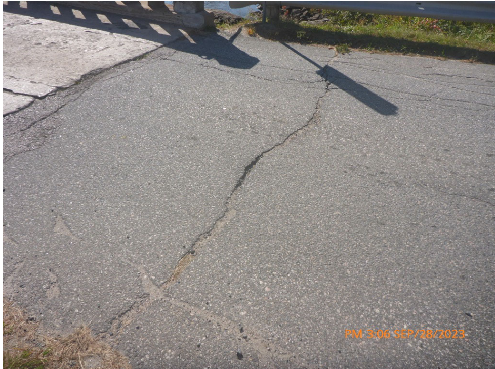
Comments: WIDE TRANSVERSE CRACK APPROACH
