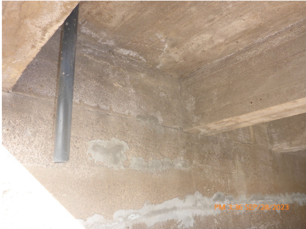
Comments: SEPARATION OF DECK AT NORTH ABUTMENT Path: P:\McKellar\2023\P1080306.jpg
