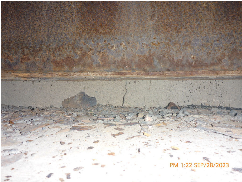
Comments: WIDE VERTICAL CRACK NORTH BALLAST WALL Path: P:\McKellar\2023\P1080230.jpg
