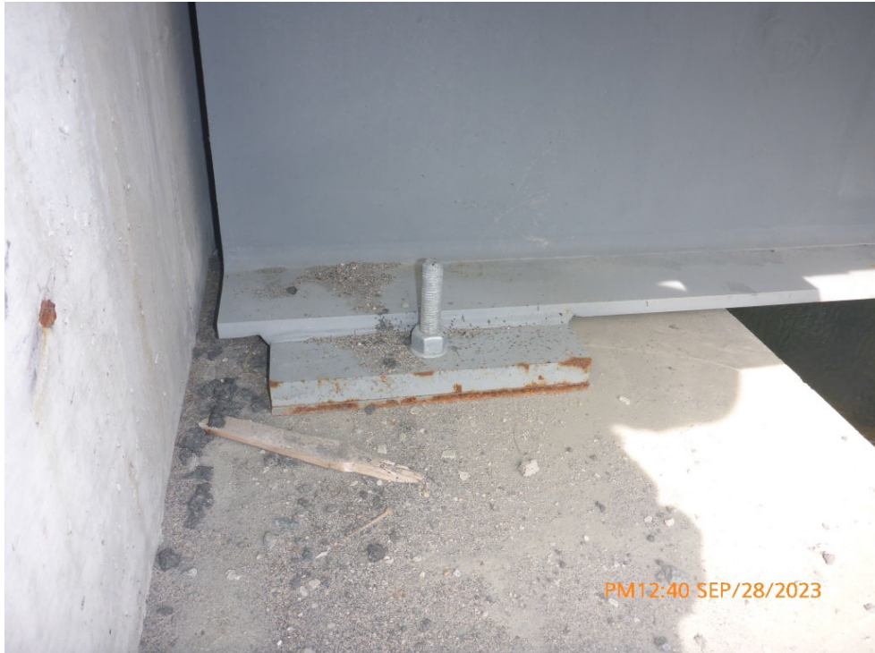
Comments: TYPICAL ABUTMENT BEARING Path: P:\McKellar\2023\P1080198.jpg
