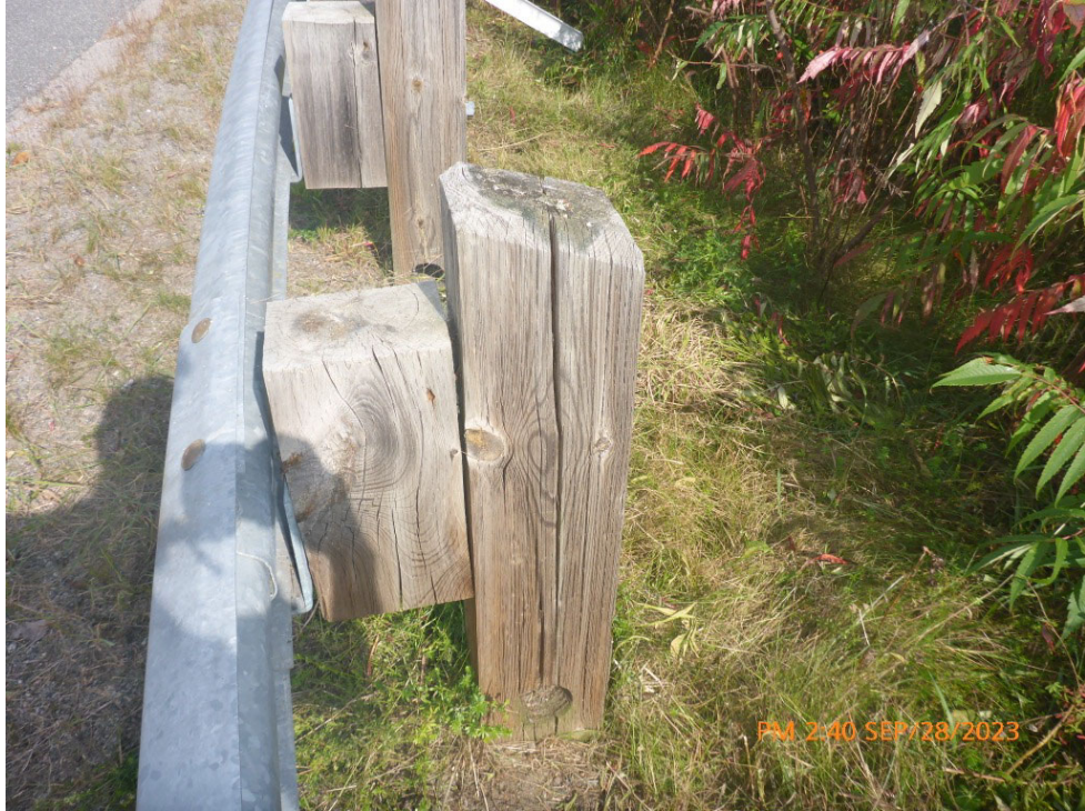
Comments: MEDIUM CHECK IN TIMBER GUIDE RAIL POST
