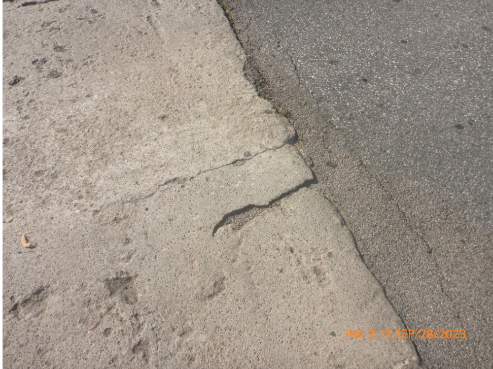
Comments: DELAMINATION NORTH END OF CONCRETE DECK
