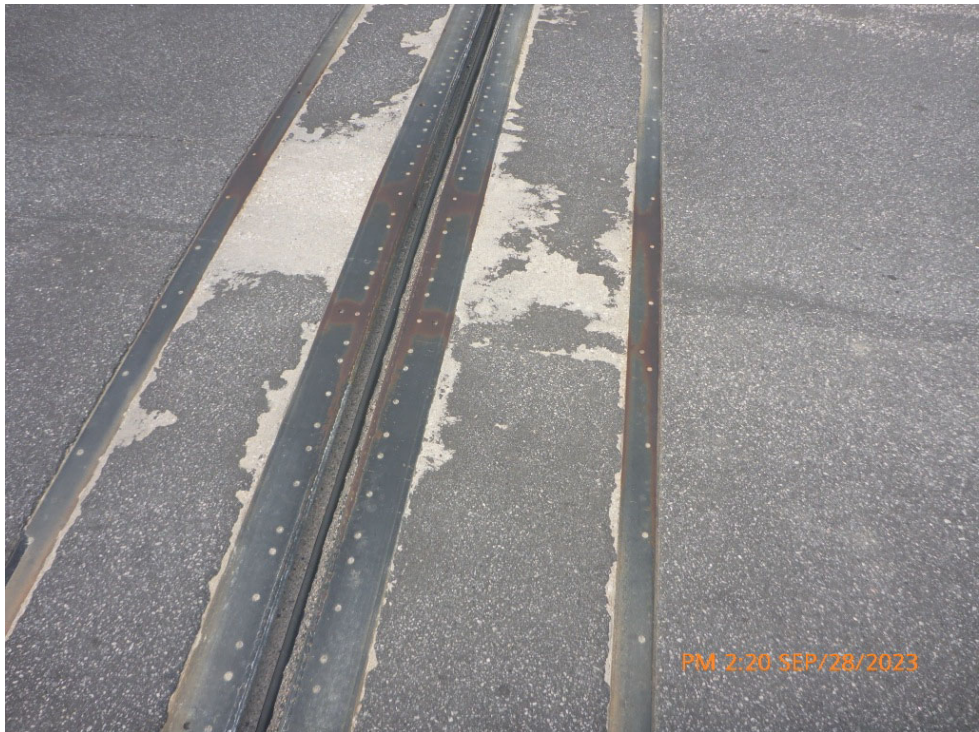
Comments: LIGHT CORROSION OF ARMOURING ANGLE
