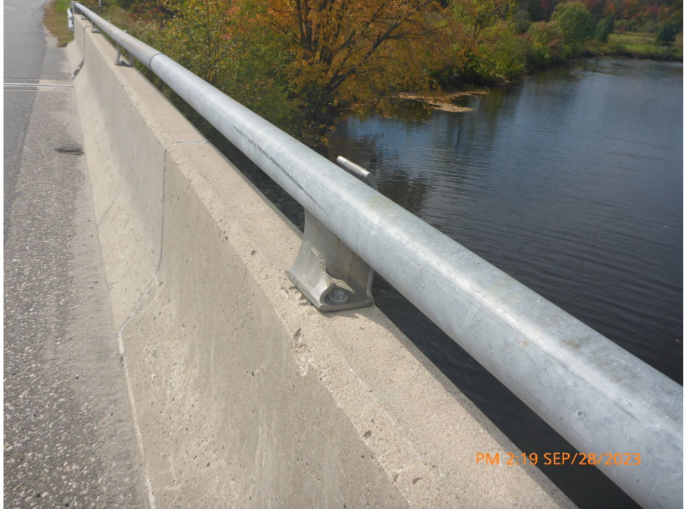
Comments: COLLISION DAMAGE TO HANDRAIL POST Path: P:\McKellar\2023\P1080242.jpg
