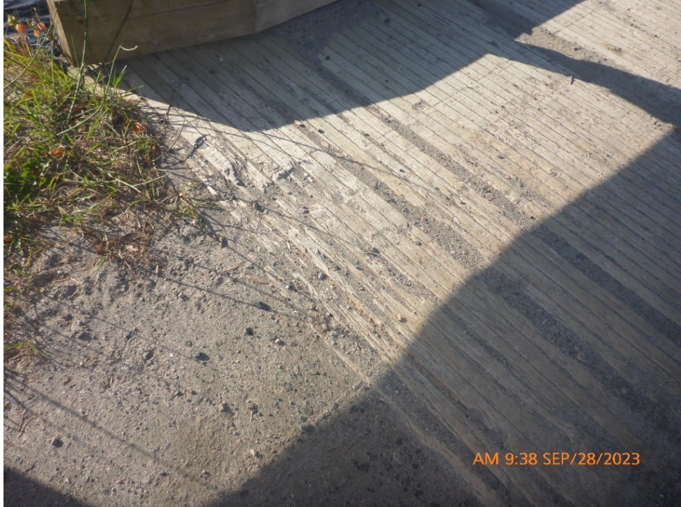
Comments: SEVERE WEATHERING OF TIMBER DECK MEMBERS
