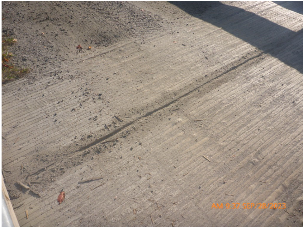
Comments: LOCALIZED SEVERE ROT OF TIMBER DECK MEMBER
