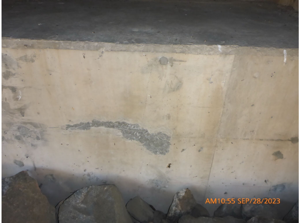
Comments: NARROW VERTICAL CRACK EAST ABUTMENT Path: P:\McKellar\2023\P1080151.jpg
