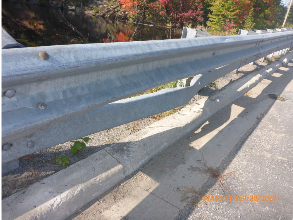
Comments: COLLISION DAMAGE APPROACH GUIDE RAIL
