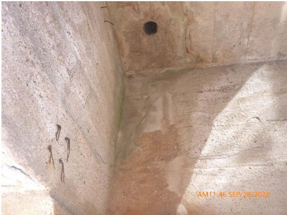
Comments: WIDE VERTICAL CRACK WEST ABUTMENT
