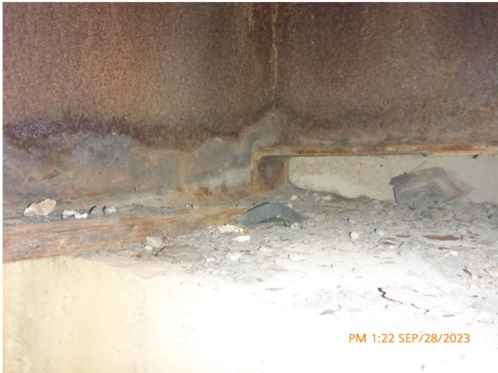
Comments: DISPLACED ELASTOMERIC BEARING PAD NORTH ABUTMENT Path: P:\McKellar\2023\P1080231.jpg
