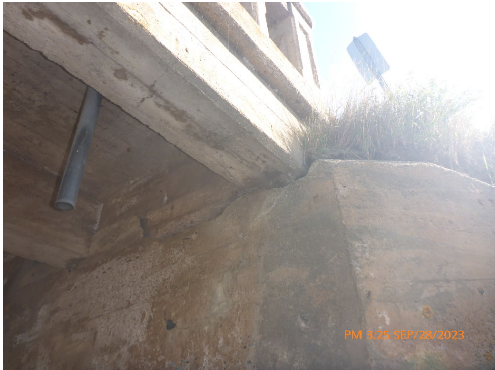
Comments: LOSS OF BEARING SURFACE BELOW EXTERIOR GIRDER SOUTH ABUTMENT Path: P:\McKellar\2023\P1080301.jpg
