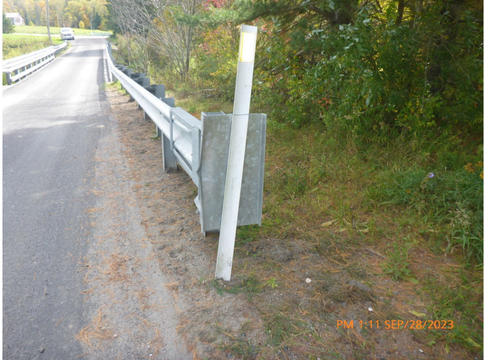
Comments: MISSING END TREATMENT HAZARD MARKER NW QUADRANT Path: P:\McKellar\2023\P1080208.jpg
