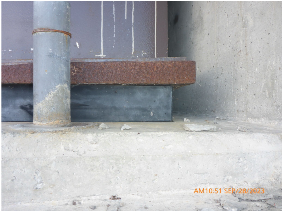
Comments: MINOR LOSS OF CONTACT ABUTMENT BEARING Path: P:\McKellar\2023\P1080146.jpg
