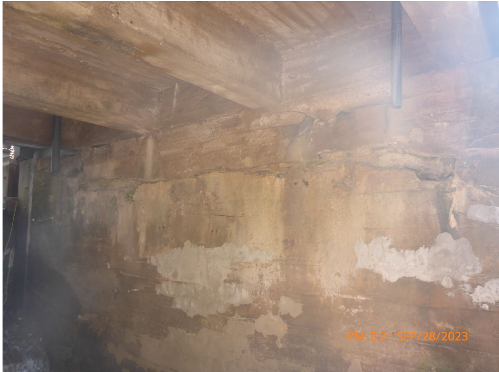
Comments: SEVERE DELAMINATIONS PIER
