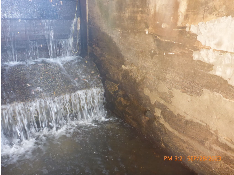
Comments: SEVERE SCOURING OF PIER Path: P:\McKellar\2023\P1080292.jpg
