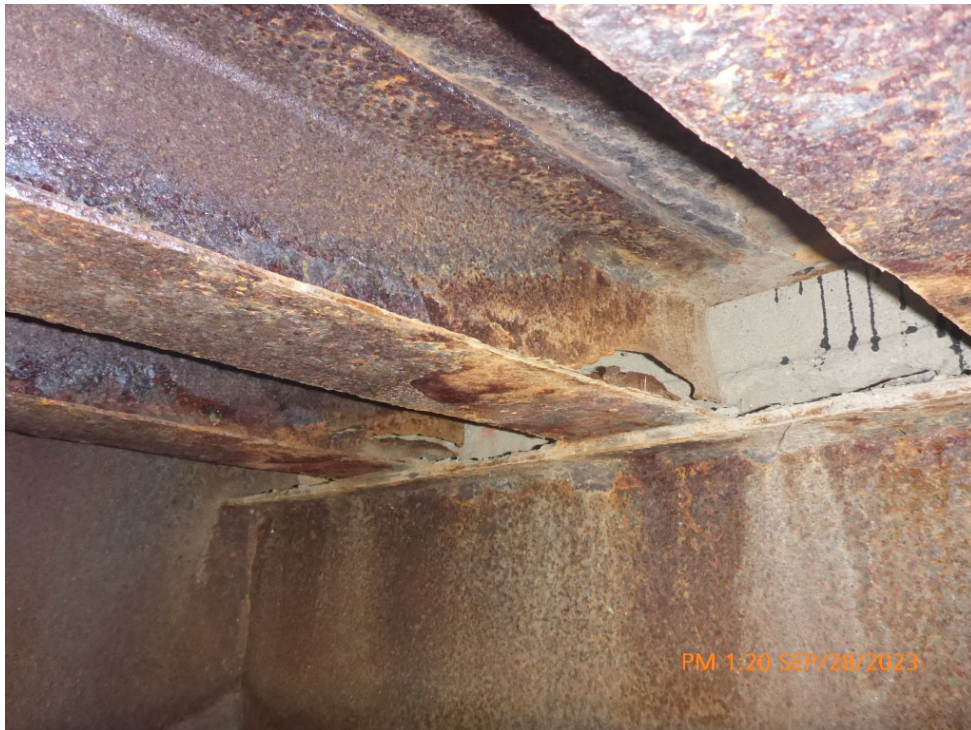
Comments: SEVERE CORROSION WITH SECTION LOSS FLOOR BEAM NORTH ABUTMENT Path: P:\McKellar\2023\P1080229.jpg
