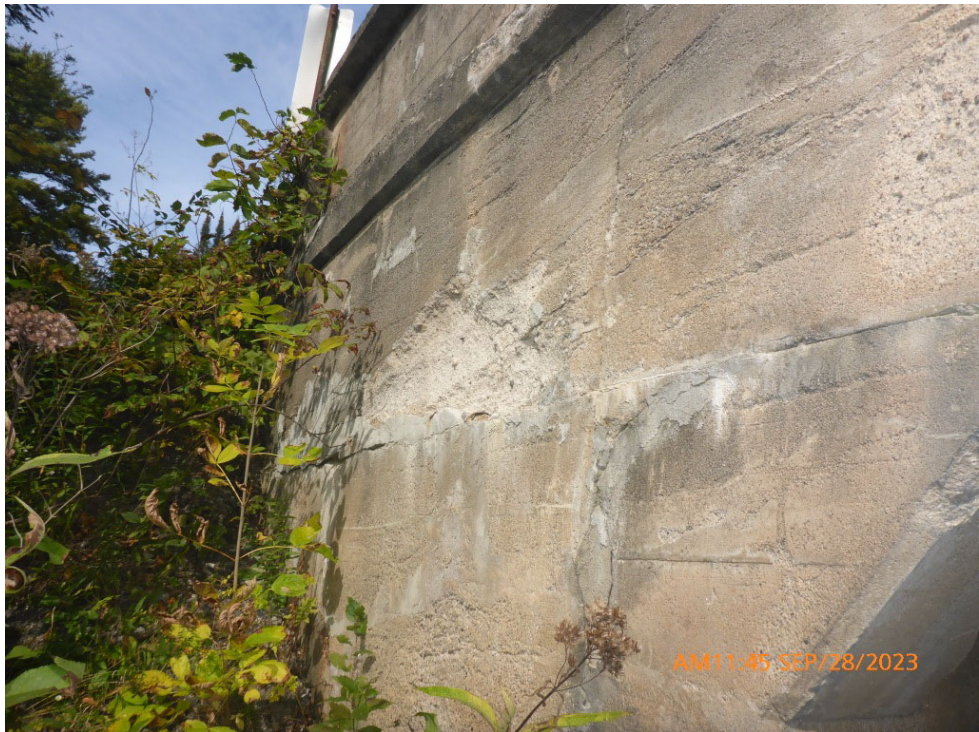
Comments: SEVERE SCALING SOUTHWEST WINGWALL
