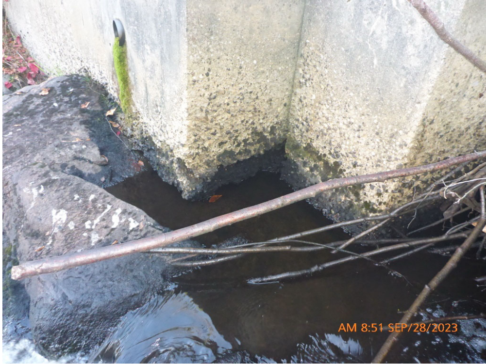
Comments: SEVERE EROSION OF CONCRETE FOOTING Path: P:\McKellar\2023\P1080090.jpg
