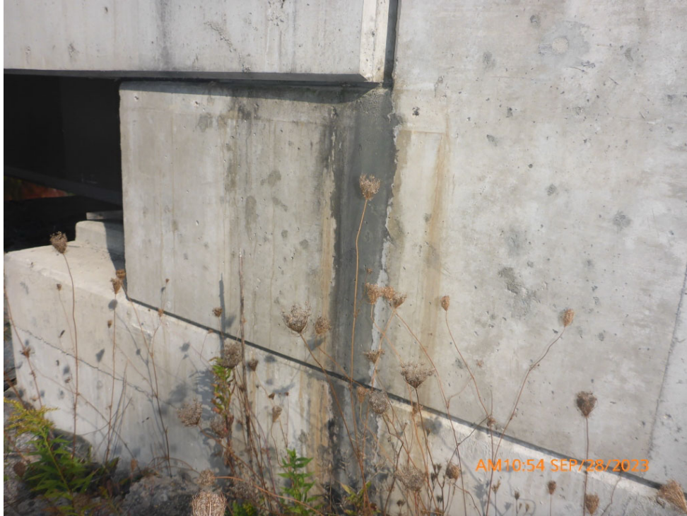
Comments: WATER STAINING ON WINGWALL
