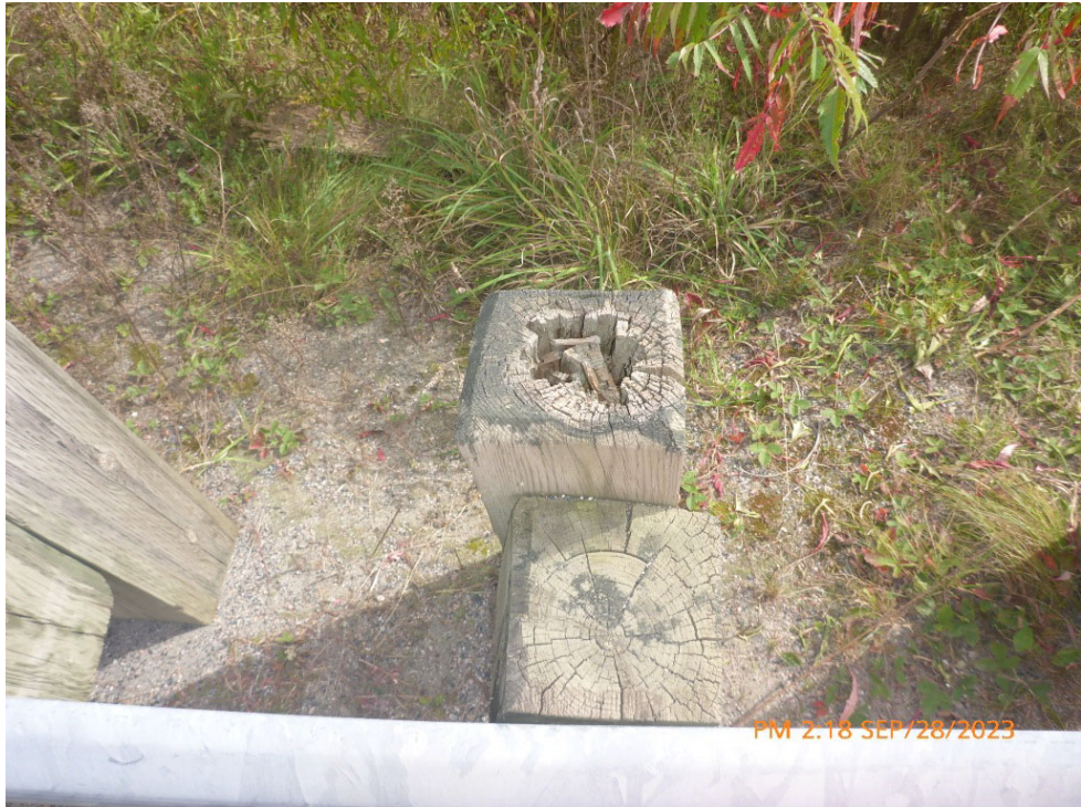
Comments: CENTRE ROT OF TIMBER GUIDE RAIL POST
