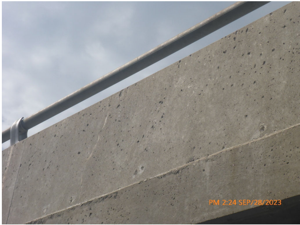
Comments: NARROW STAINED CRACK EXTERIOR PARAPET WALL Path: P:\McKellar\2023\P1080251.jpg
