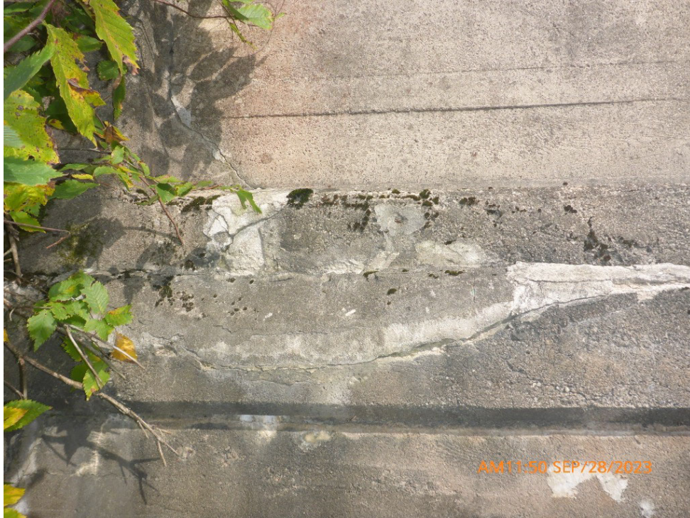
Comments: SEVERE DELAMINATION EXTERIOR FASCIA
