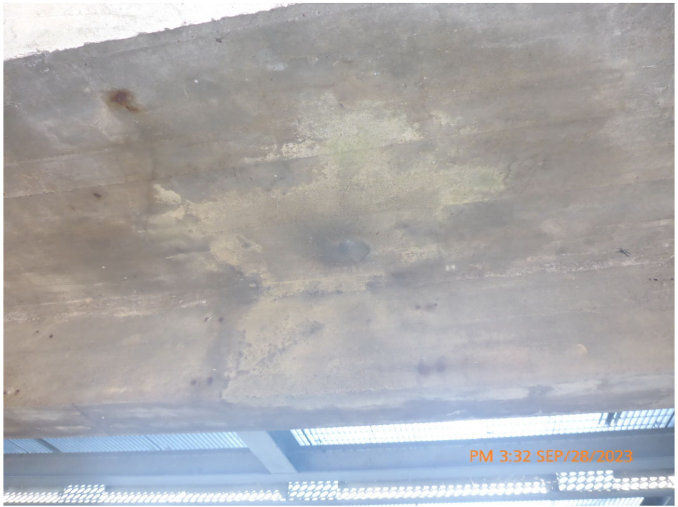
Comments: MISSING DECK DRAIN Path: P:\McKellar\2023\P1080305.jpg
