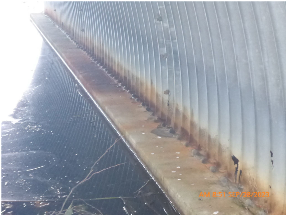
Comments: MEDIUM CORROSION OF EAST BARREL WALL AT FOOTING
