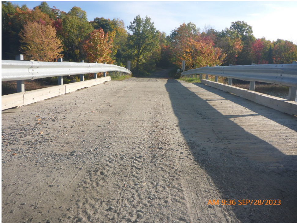
Comments: MEDIUM WHEEL TRACK RUTTING IN TIMBER DECK
