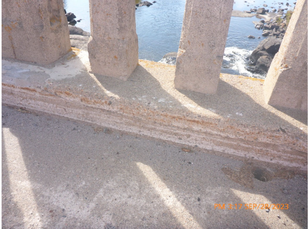
Comments: DELAMINATION IN CONCRETE CURB
