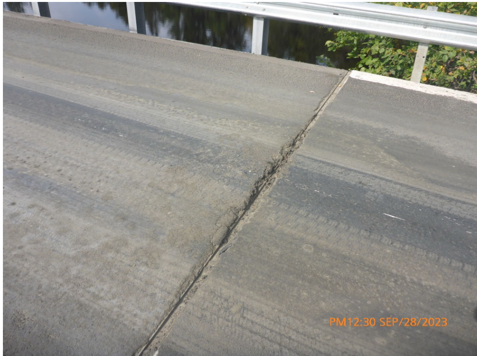
Comments: MINOR DETERIORATION OF ASPHALT AT DECK END Path: P:\McKellar\2023\P1080188.jpg
