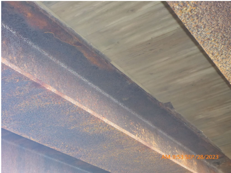
Comments: SEVERE FLAKING OF STEEL GIRDER FLANGE Path: P:\McKellar\2023\P1080122.jpg
