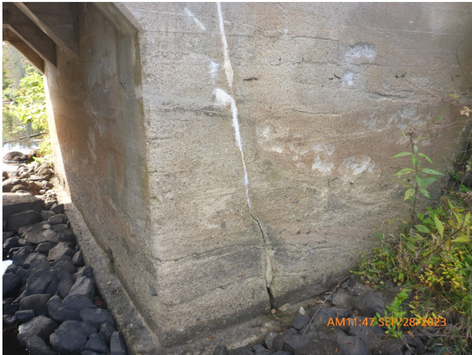
Comments: WIDE VERTICAL CRACK NORTHWEST WINGWALL
