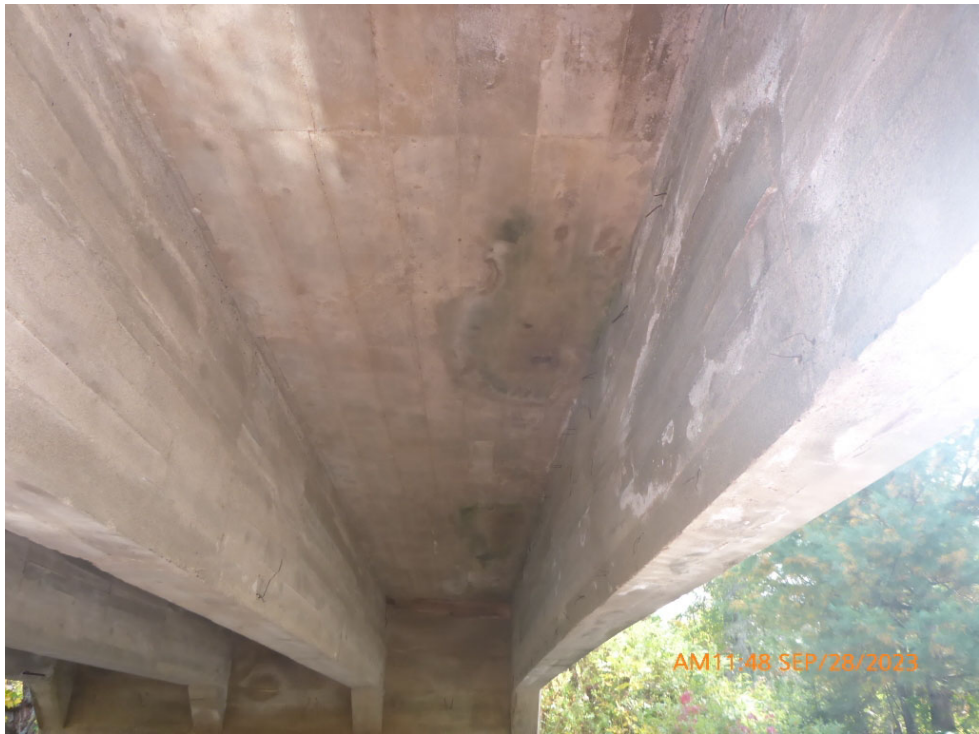
Comments: WATER STAINING INTERIOR SOFFIT Path: P:\McKellar\2023\P1080180.jpg
