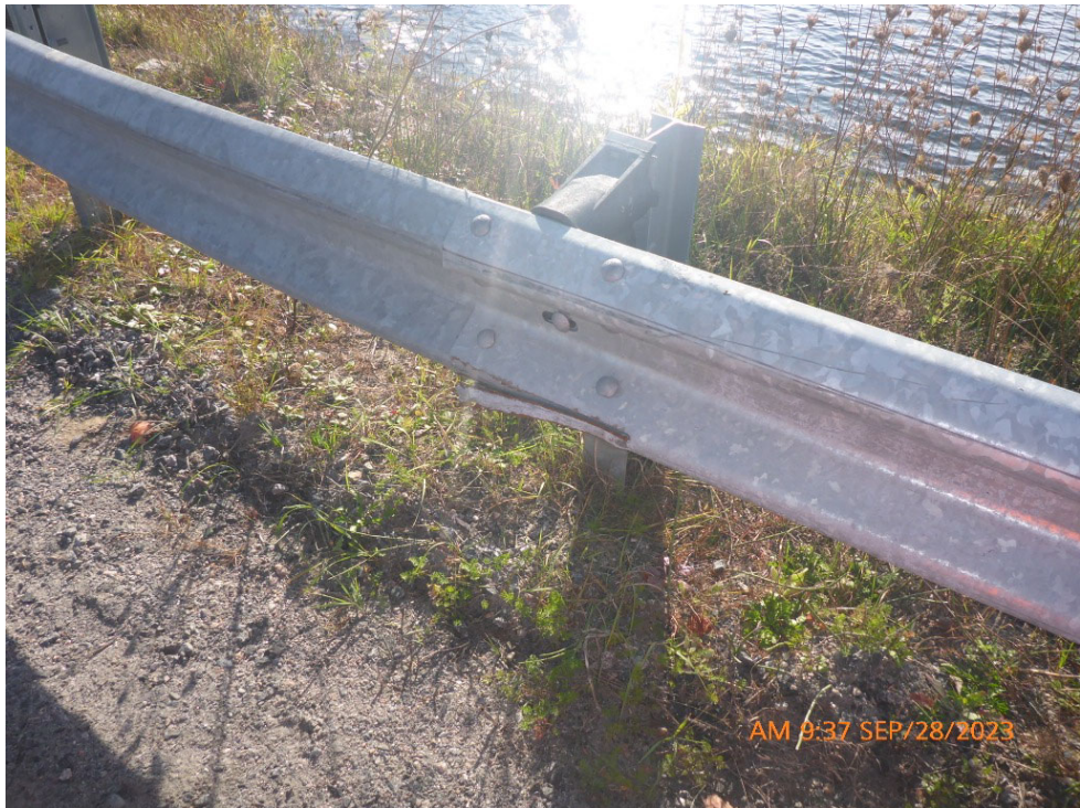
Comments: TEAR IN GUIDE RAIL ON APPROACH
