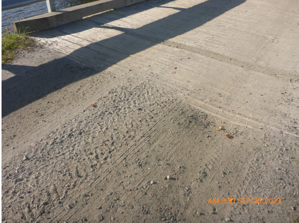
Comments: LIGHT POTHOLE IN EAST APPROACH
