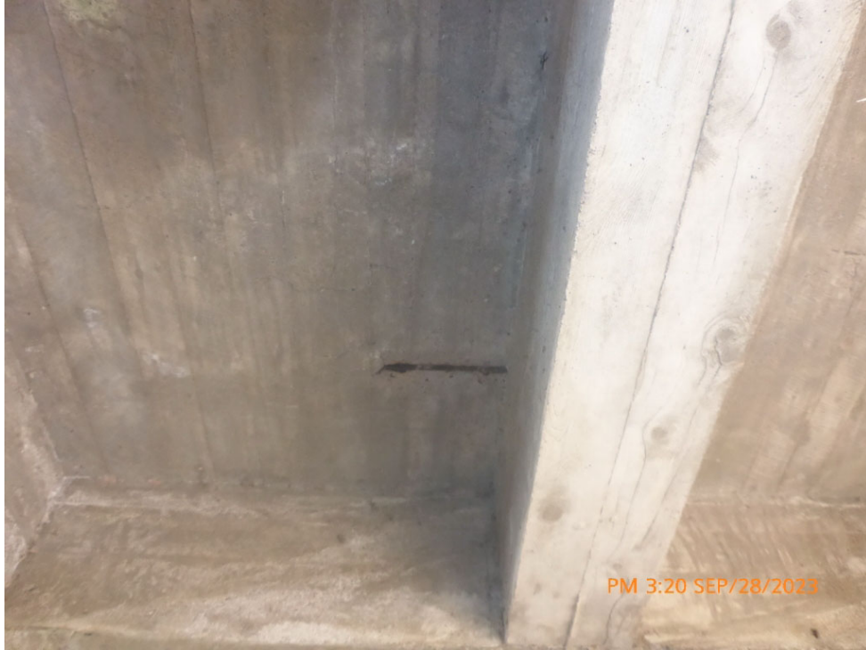
Comments: SPALLING INTERIOR SOFFIT Path: P:\McKellar\2023\P1080289.jpg
