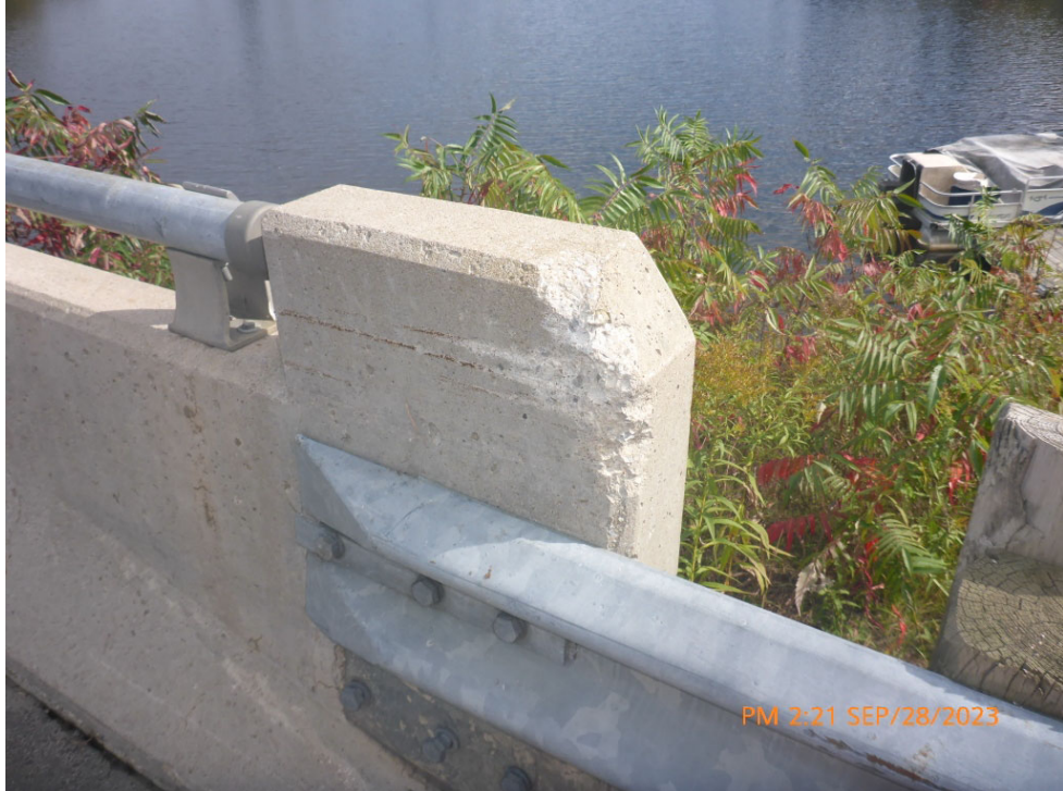
Comments: LIGHT ABRASION PARAPET END POST
