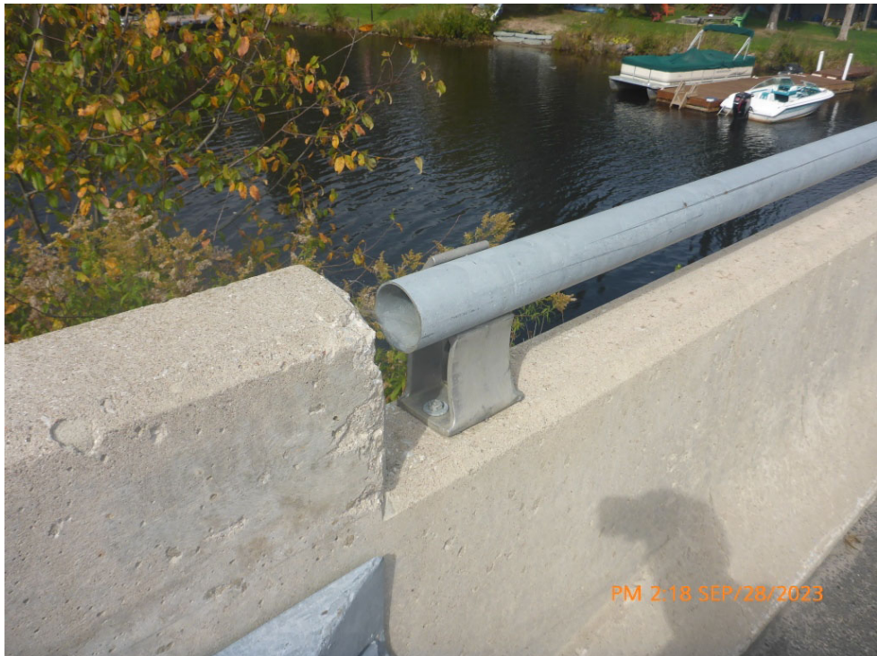
Comments: MISSING END CAP SOUTHWEST QUADRANT
