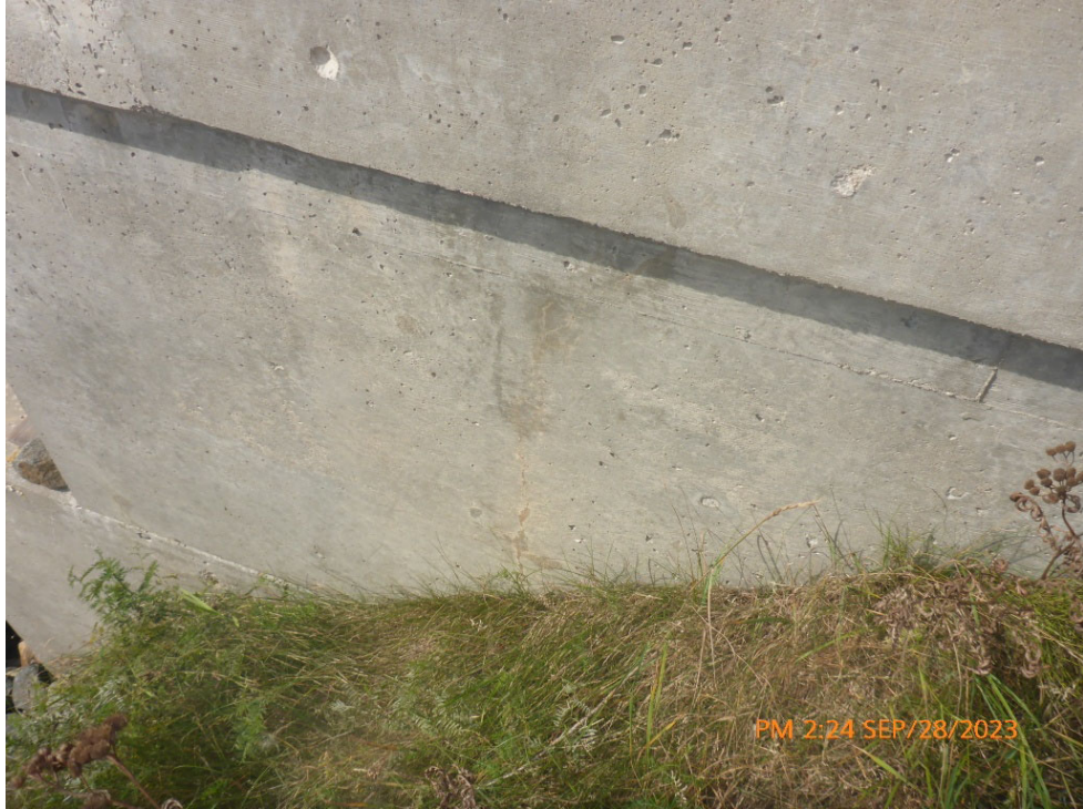
Comments: NARROW STAINED CRACK IN WINGWALL
