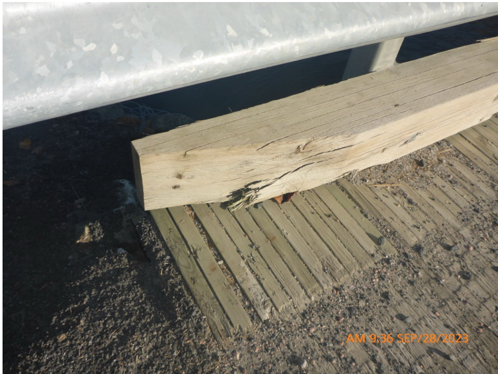
Comments: MINOR ABRASION IN TIMBER CURB
