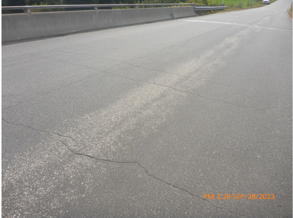
Comments: NARROW CRACKS IN DECK WEARING SURFACE
