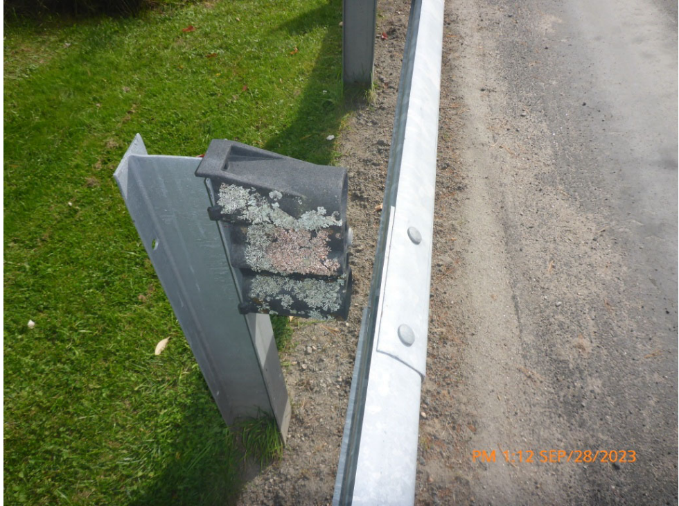
Comments: GUIDE RAIL DISCONNECTED GUIDE RAIL NORTH APPROACH
