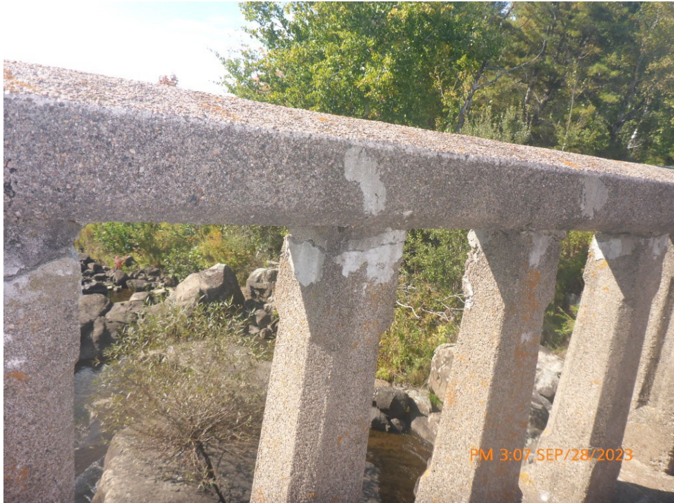
Comments: WIDE CRACKS IN BALUSTRADE
