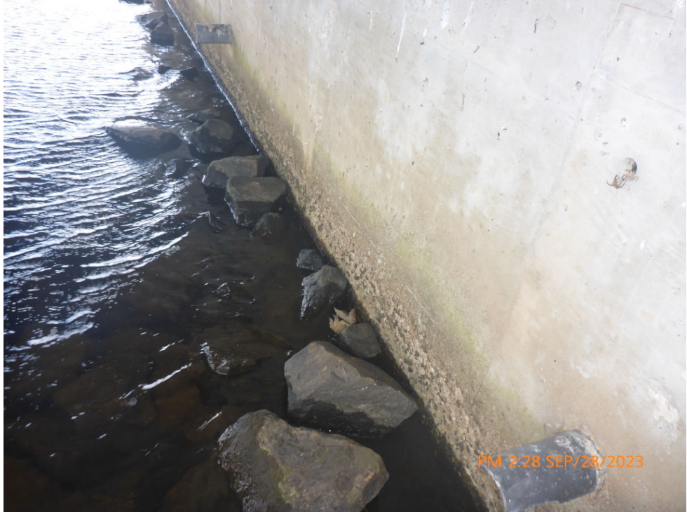
Comments: LIGHT EROSION OF SOUTH ABUTMENT AT WATERLINE Path: P:\McKellar\2023\P1080258.jpg
