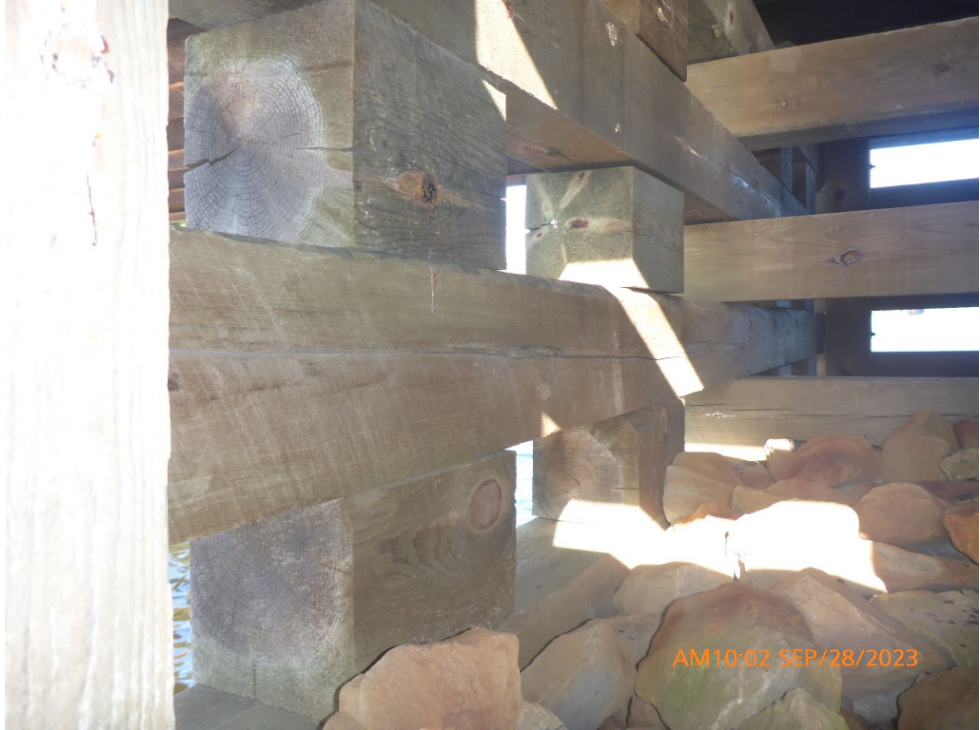
Comments: SEVERE CHECK IN TIMBER CRIB MEMBER Path: P:\McKellar\2023\P1080124.jpg
