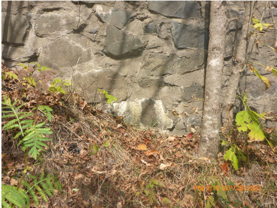
Comments: EFFLORESCENT STAINING NORTHWEST WINGWALL
