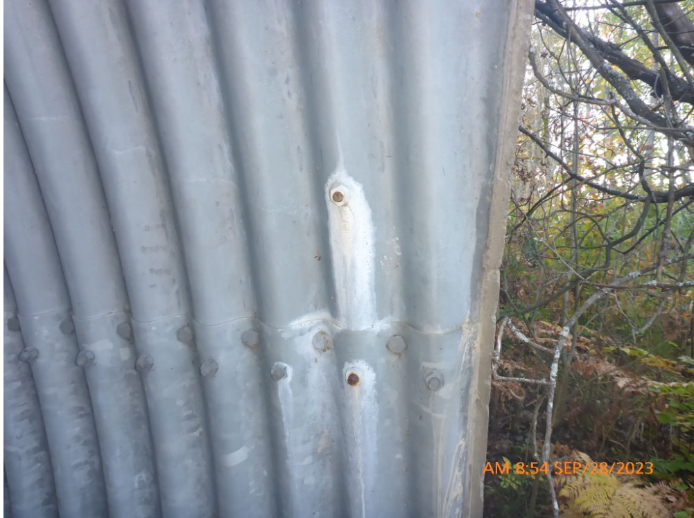
Comments: ENCRUSTATION AT BOLT LOCATION
