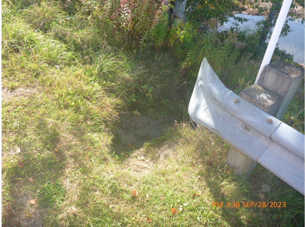
Comments: SEVERE EROSION OF ROADWAY EMBANKMENT SOUTHWEST QUADRANT
