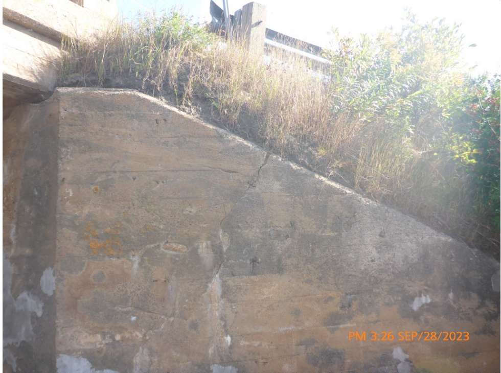
Comments: WIDE VERTICAL CRACK IN WINGWALL
