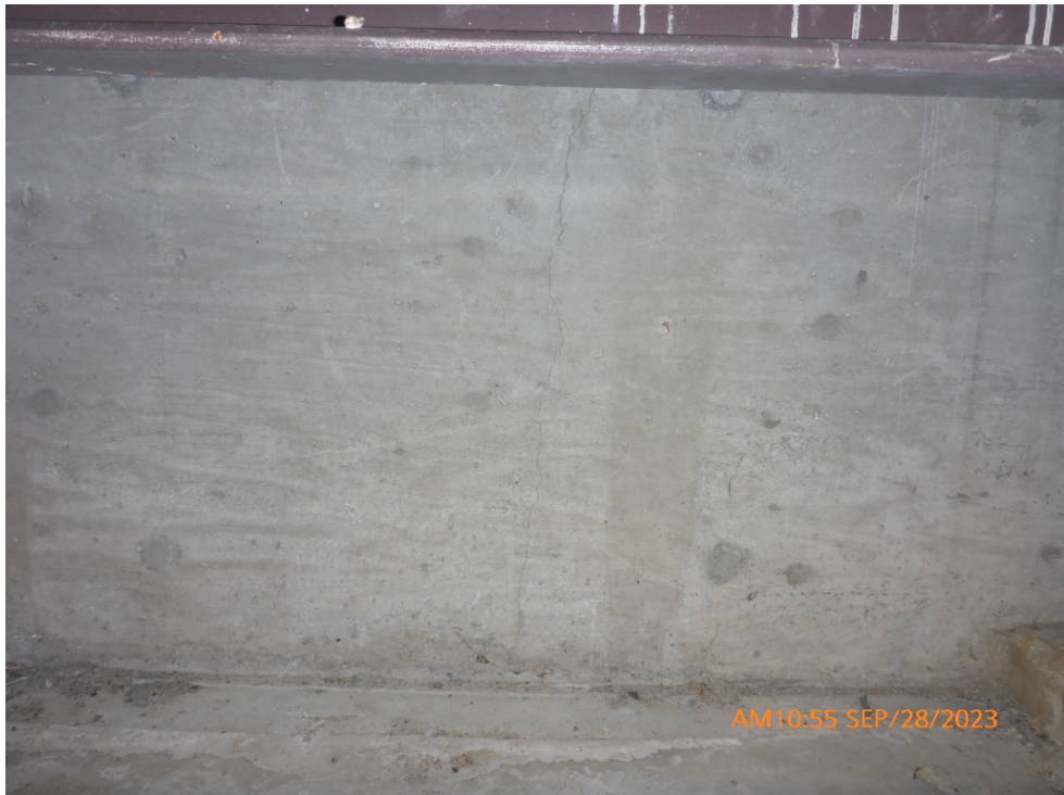
Comments: NARROW VERTICAL CRACK EAST BALLAST WALL Path: P:\McKellar\2023\P1080152.jpg
