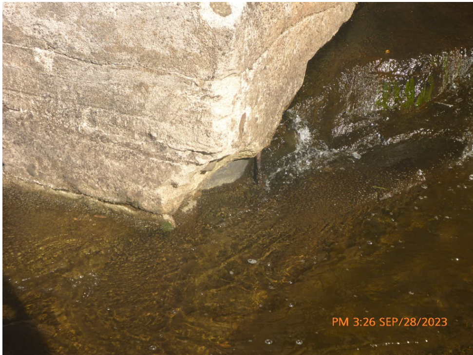
Comments: SEVERE SCOURING OF PIER AT WATERLINE Path: P:\McKellar\2023\P1080303.jpg
