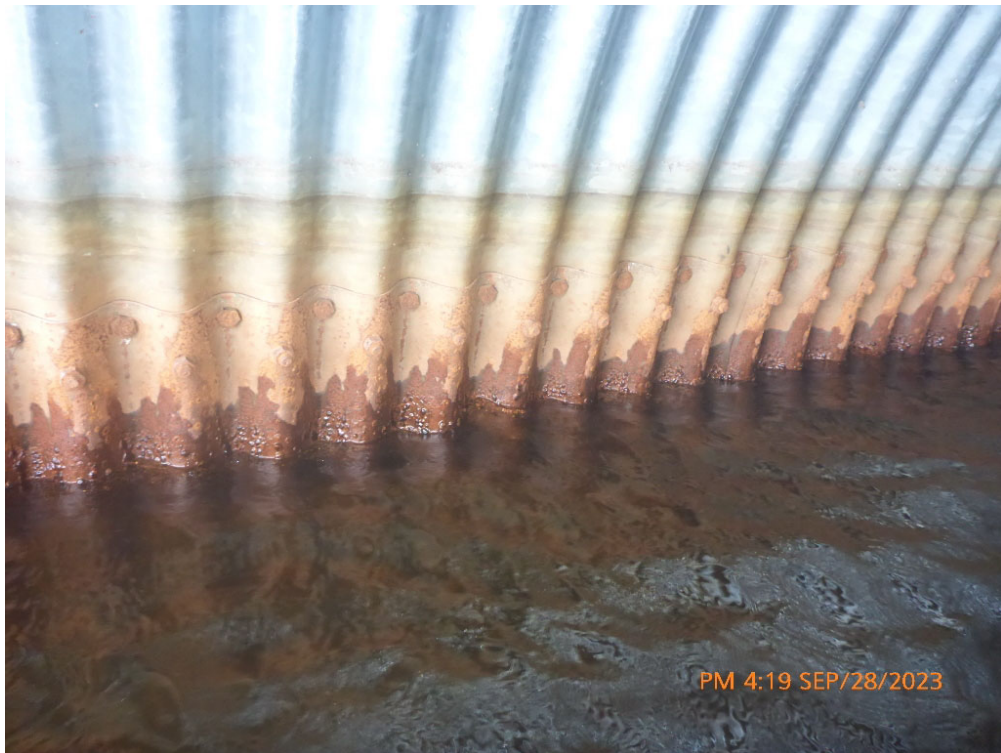
Comments: LIGHT CORROSION OF BARREL AT WATERLINE Path: P:\McKellar\2023\P1080315.jpg
