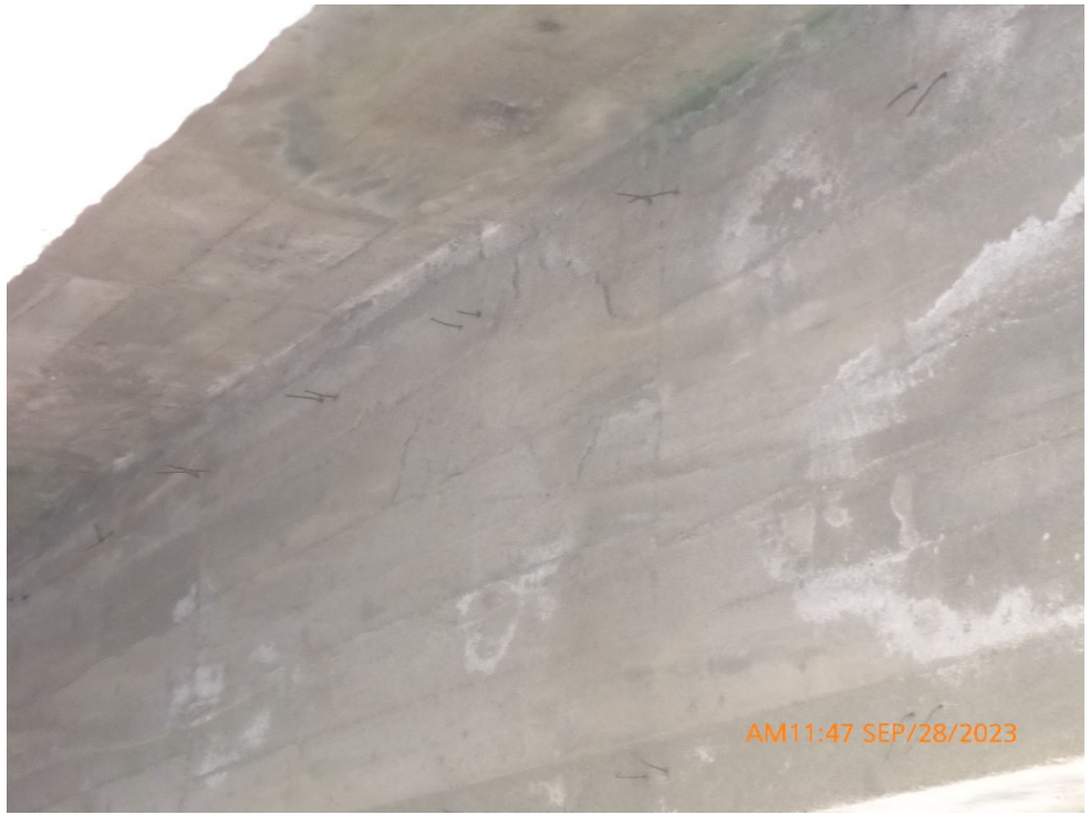
Comments: SEVERE DELAMINATION T-BEAM GIRDER
