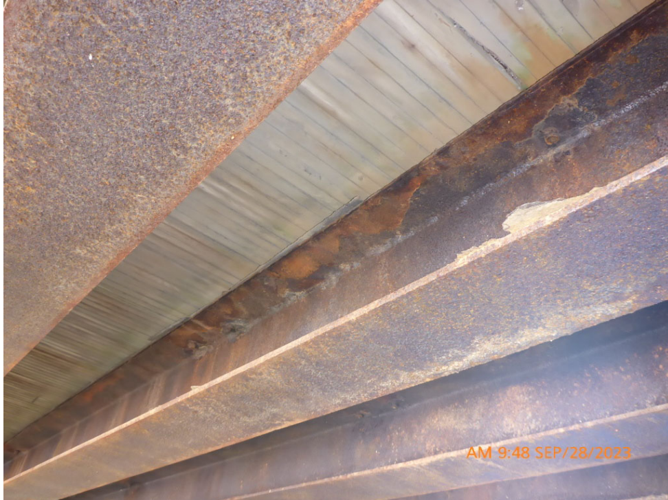
Comments: SEVERE FLAKING OF STEEL GIRDER FLANGE Path: P:\McKellar\2023\P1080117.jpg
