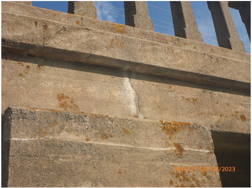
Comments: WIDE CRACK IN EXTERIOR FASCIA
