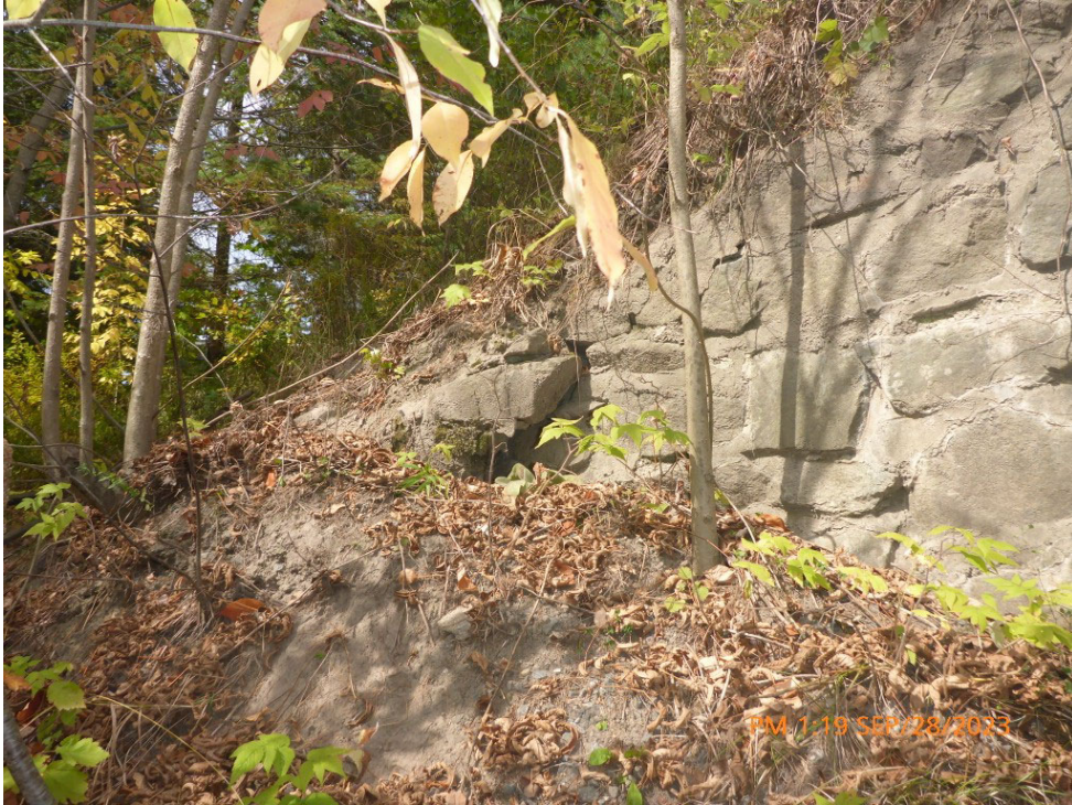
Comments: BROKEN SECTION OF NORTHWEST WINGWALL
