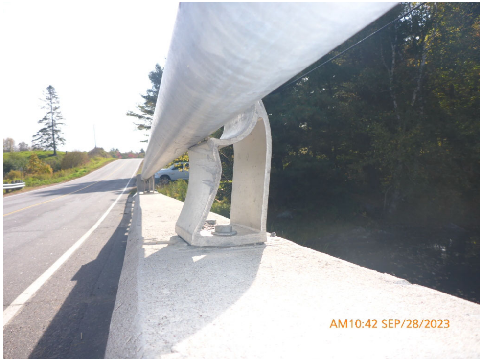
Comments: MISSING BOLT PARAPET HAND RAILING Path: P:\McKellar\2023\P1080134.jpg
