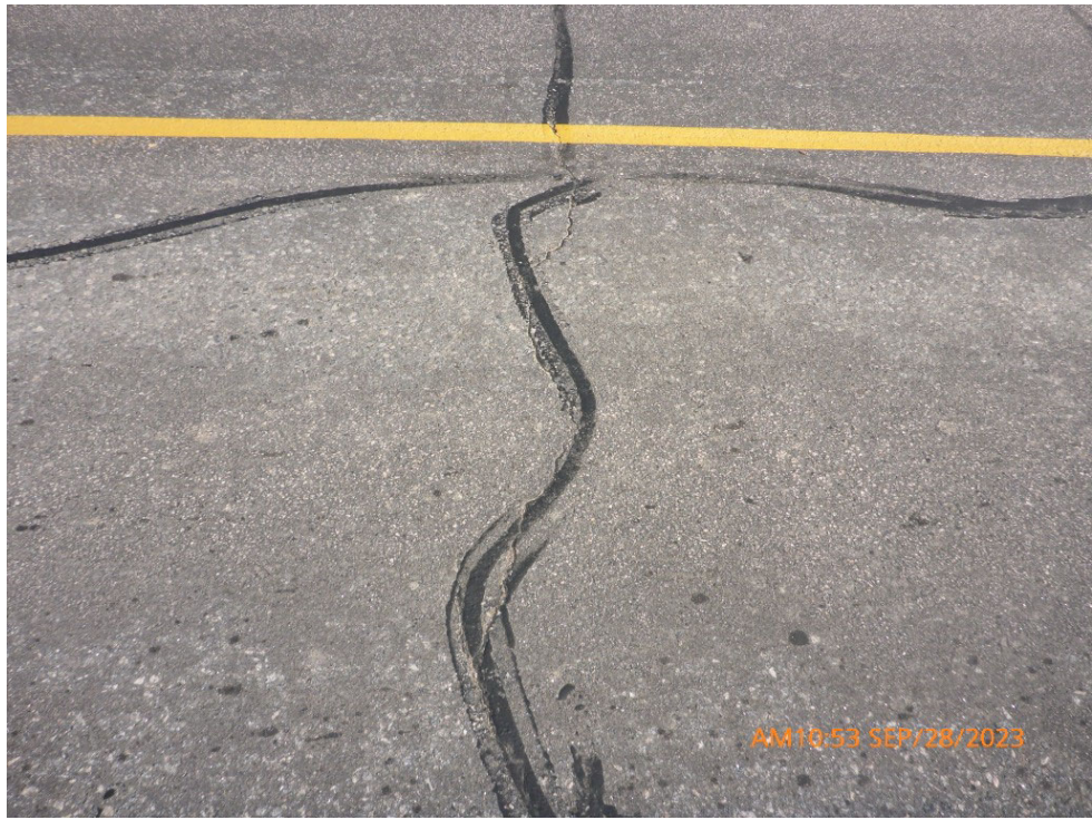
Comments: NARROW TRANSVERSE CRACK IN WEARING SURFACE Path: P:\McKellar\2023\P1080149.jpg
