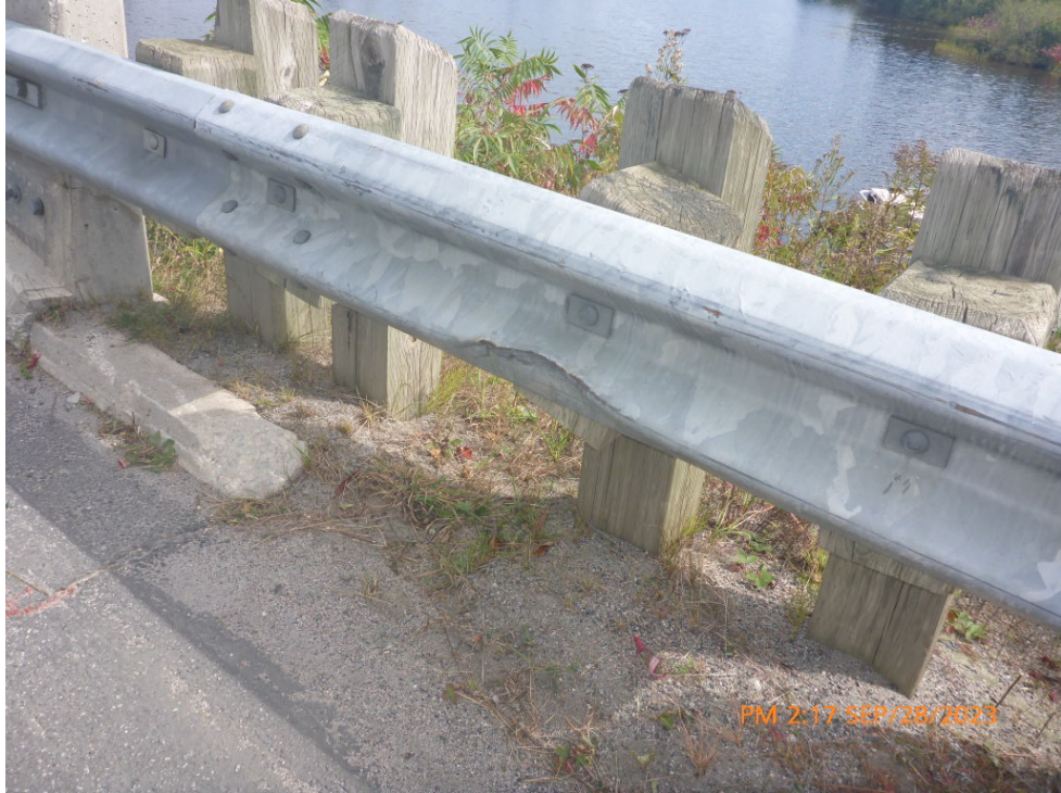
Comments: COLLISION DAMAGE APPROACH GUIDE RAIL
