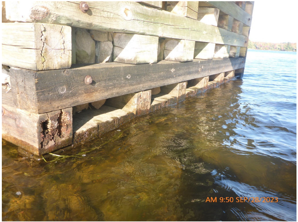
Comments: MEDIUM ROT OF TIMBER CRIB MEMBERS WEST ABUTMENT
