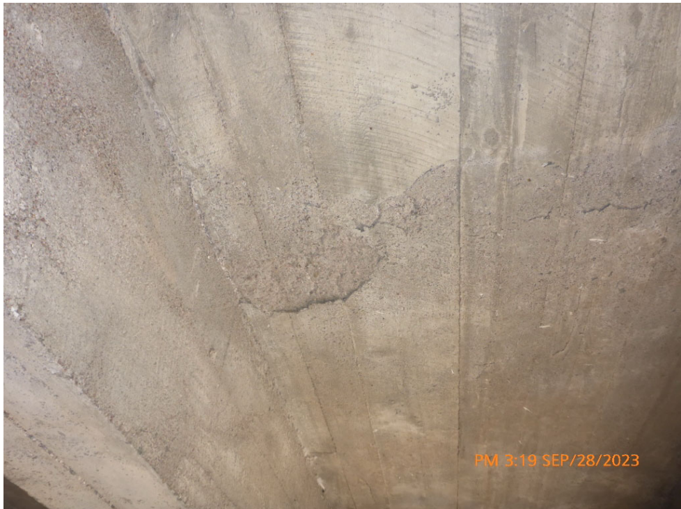
Comments: DELAMINATION INTERIOR SOFFIT
