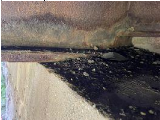
Photo 3: Severe corrosion and section loss of girder flange near bearing.
