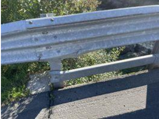
Photo 1: Impact damage at south end of west guiderail
