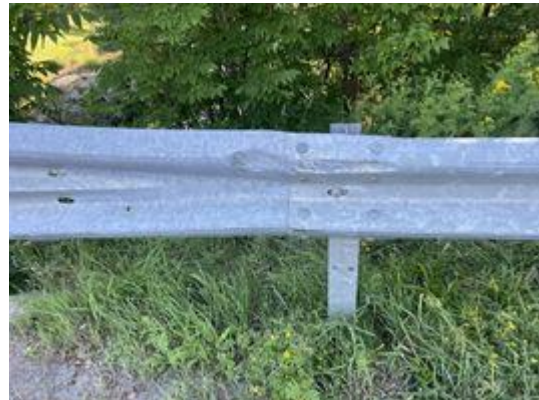
Photo 2: Impact damage to the south end of the northwest guiderail
