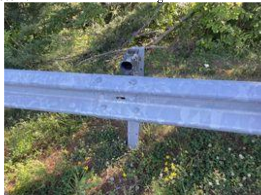
Photo 4: Post disconnected from guiderail
