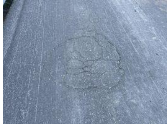
Photo 2: Circular depression with light alligator cracking
