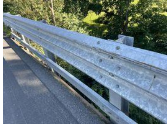
Photo 2: Abrasion and light corrosion at top of guiderail
