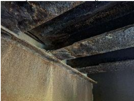
Photo 3: Very severe corrosion at stringer ends
