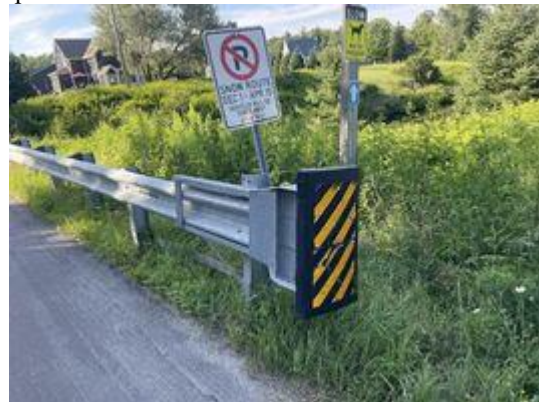
Photo 2: Abrasion and tears in south hazard sign, no snowplow delineator
