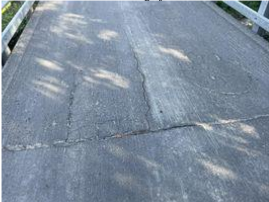
Photo 1: Medium crack at bridge joint.
