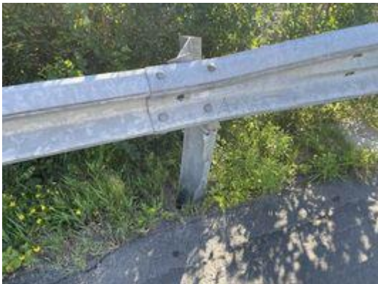
Photo 3: Damaged post at the north end of the southwest guiderail.
