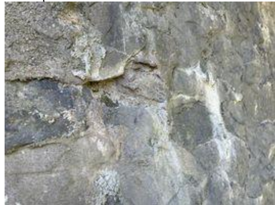
Photo 2: Spall and incrustation
