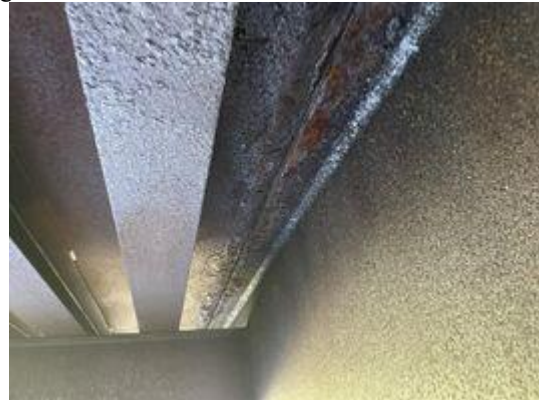
Photo 2: Moderate corrosion with section loss around top flange
