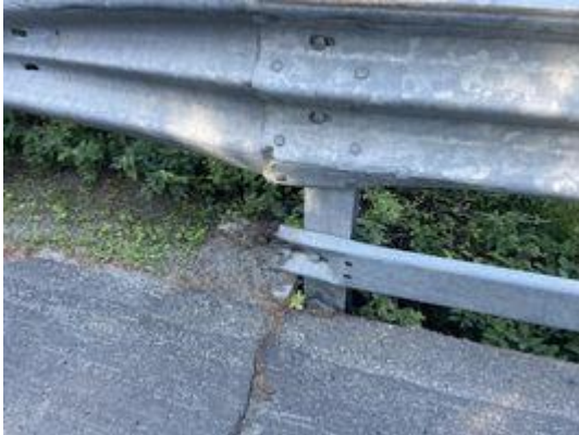
Photo 3: Impact damage to channel end
