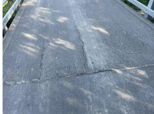
Photo 4: Light alligator cracking at north end of deck
