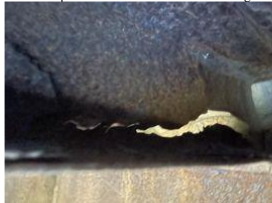
Photo 2: Complete section loss at the north stringer ends
