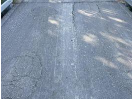
Photo 3: Wheel rutting with longitudinal cracks
