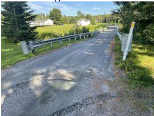
Photo 3: Hazard signs or snowplow delineators not installed at the north approach
