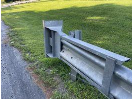
Photo 1: Northeast end treatment post is twisted
