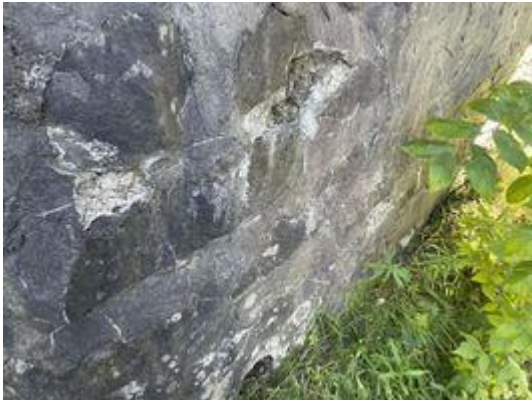
Photo 1: Light mortar loss, spall, and narrow cracks with efflorescence
