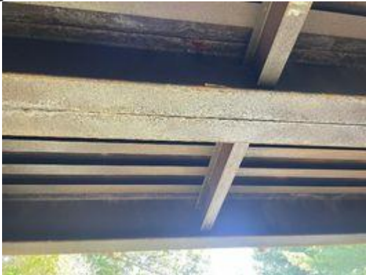
Photo 1: Moderate corrosion and flaking patina at bottom flanges
